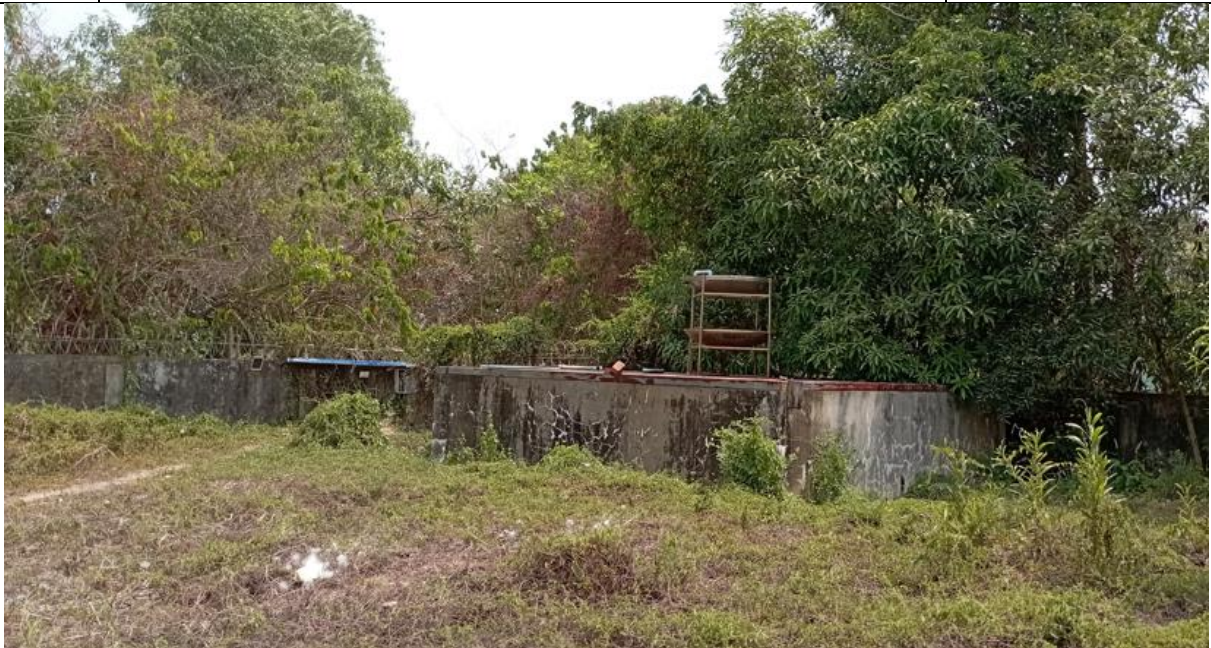
Figure 3.5.7.1: Ground water Source and Ground Water Storage Tank
