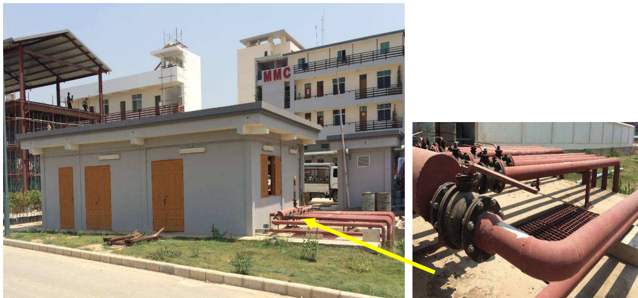
Figure 2.10 Wastewater Treatment Plant for Mingalar Mandalay Project
