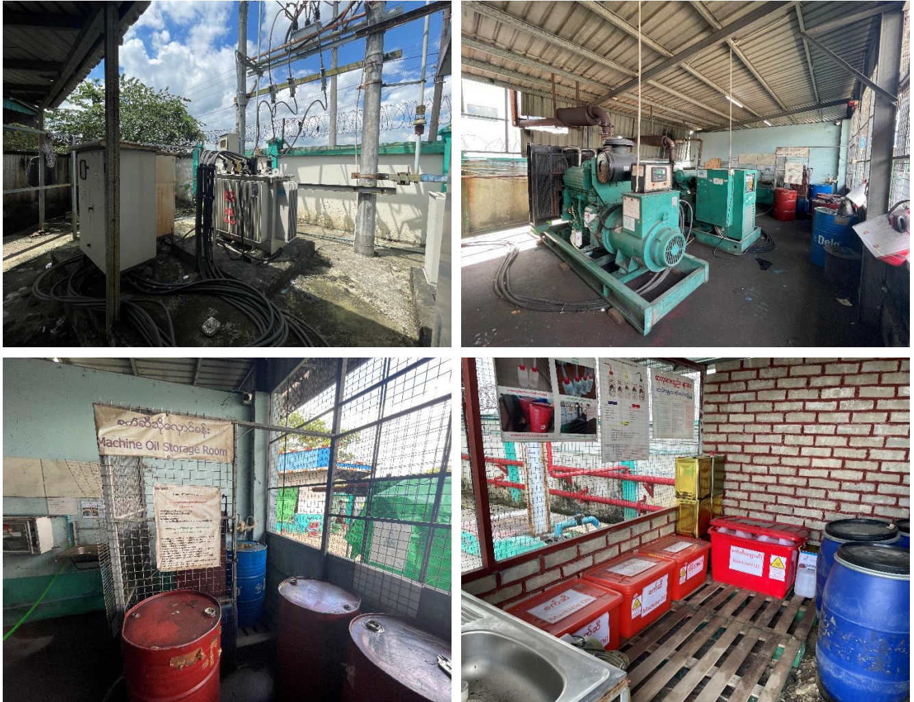
Figure 1-11 Transformer, Generator Room and Fuel Storage Area
