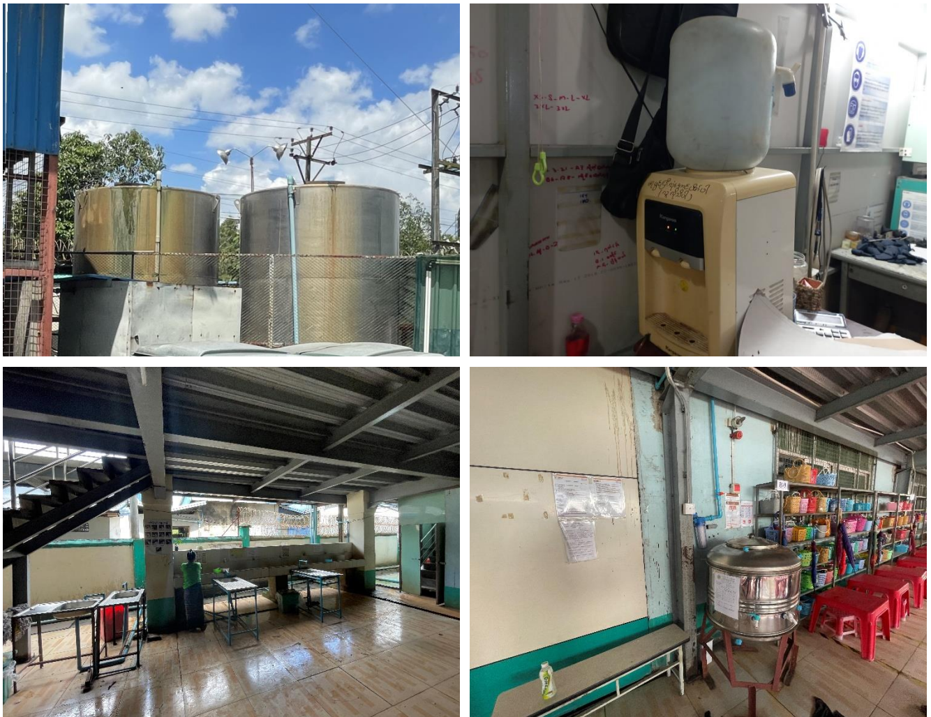
Figure 1-10 Water Storage Tank and Drinking Water Supply System
