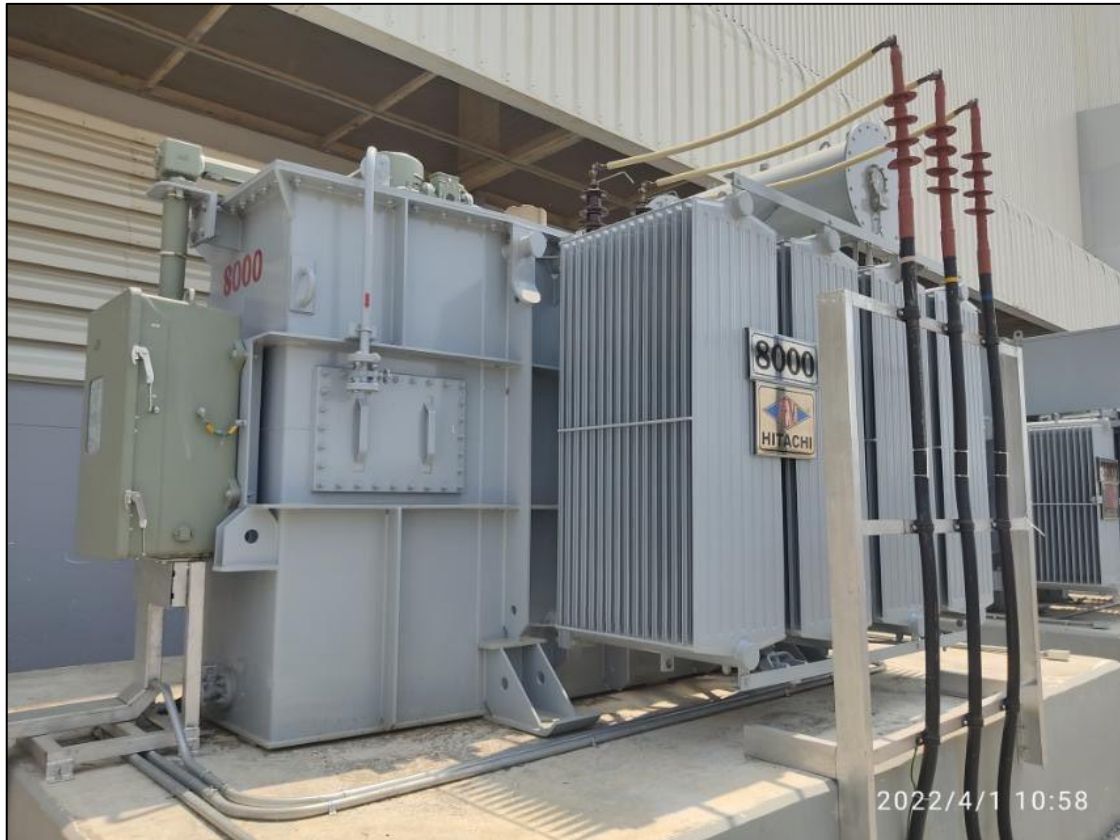
Figure 3-33 Photo of Transformer
