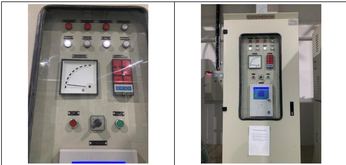
Figure 10 Photo of On Load Tap Changer
