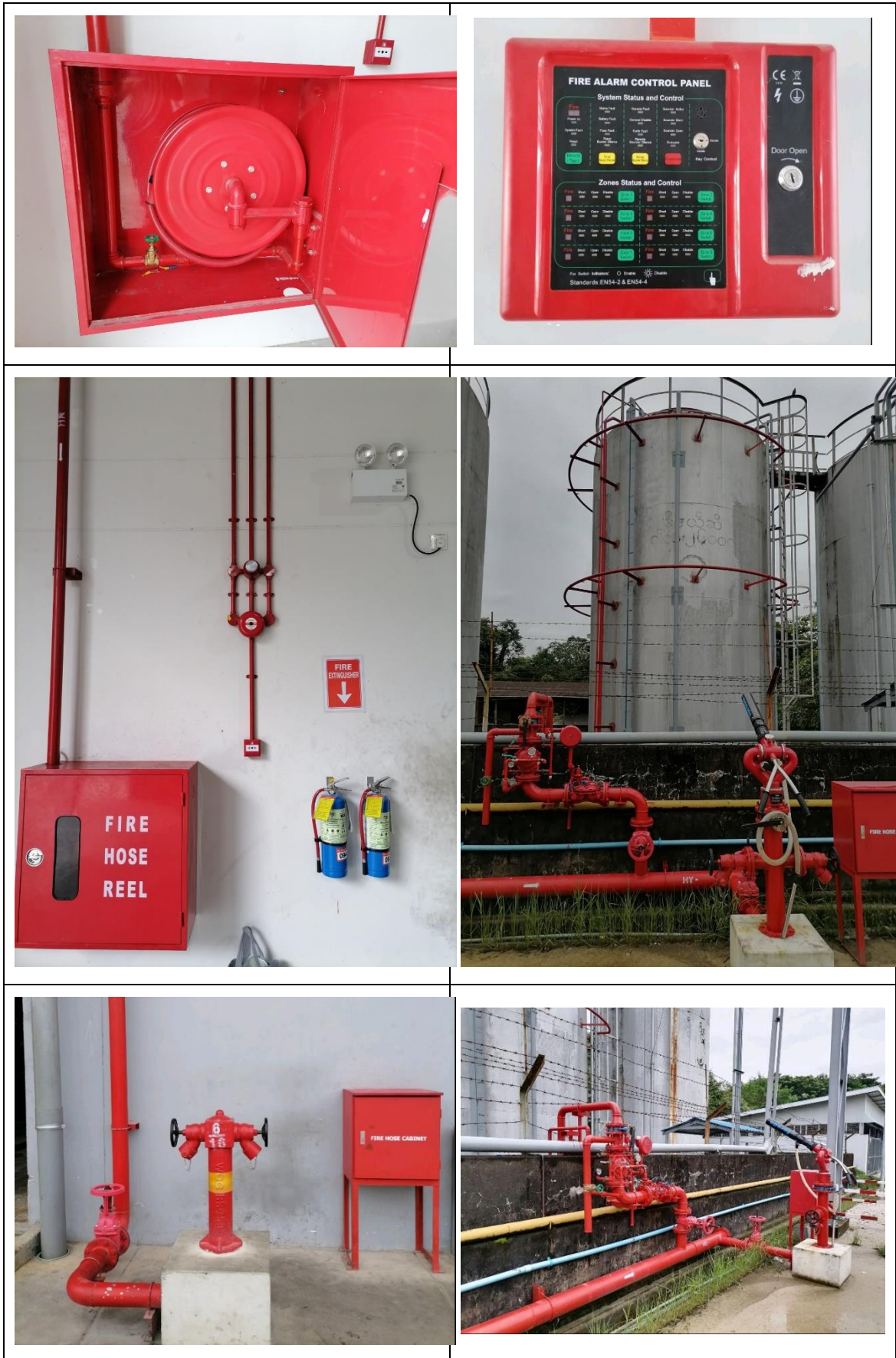
Figure 7-15 Fire Management System
