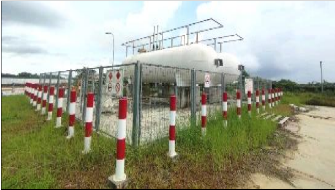
Figure 3-37 LPG Storage Tank
