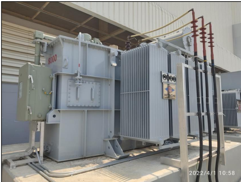
Figure 9 Photo of Transformer
