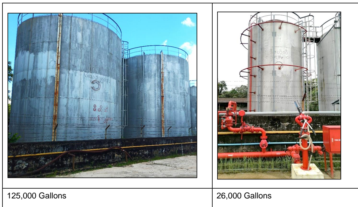
Figure 3-36 Diesel Storage Tank
