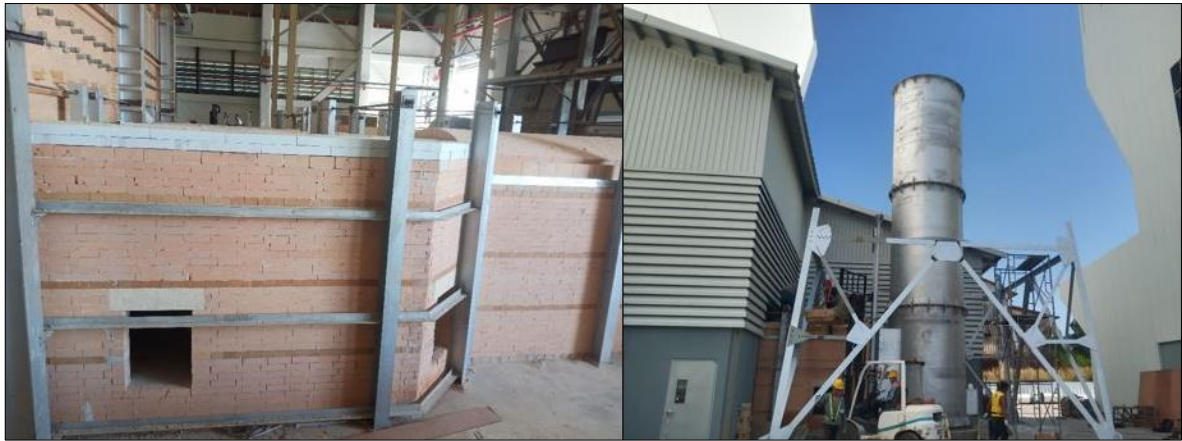
Figure 3-21 Furnace and Chimney
