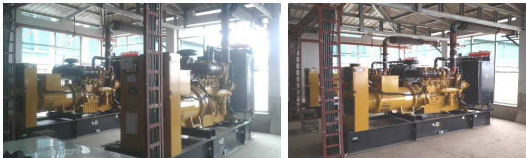
Figure 3. 6 Generators (500kVA-2 Nos)
