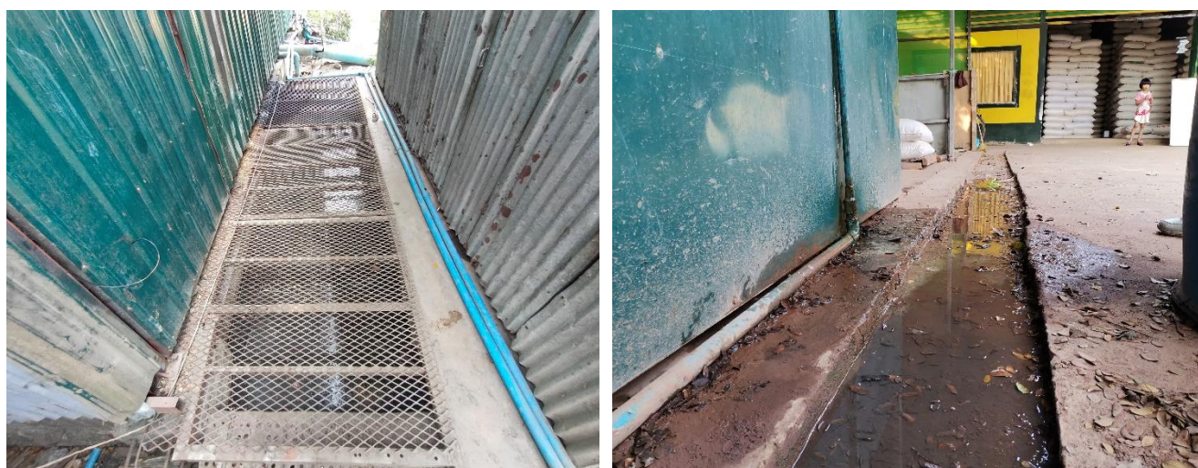
Figure 1-17 Liquid Waste Control Facility
