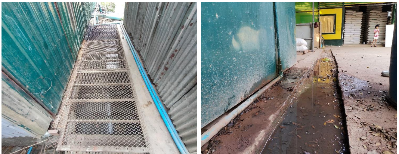
Figure 1-17 Liquid Waste Control Facility
