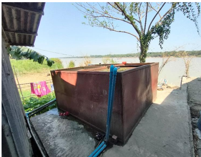
Fire fighting tank
