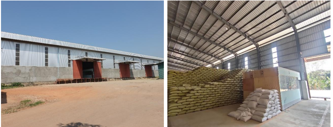
Figure 1-14 Ventilation system implementation photo
