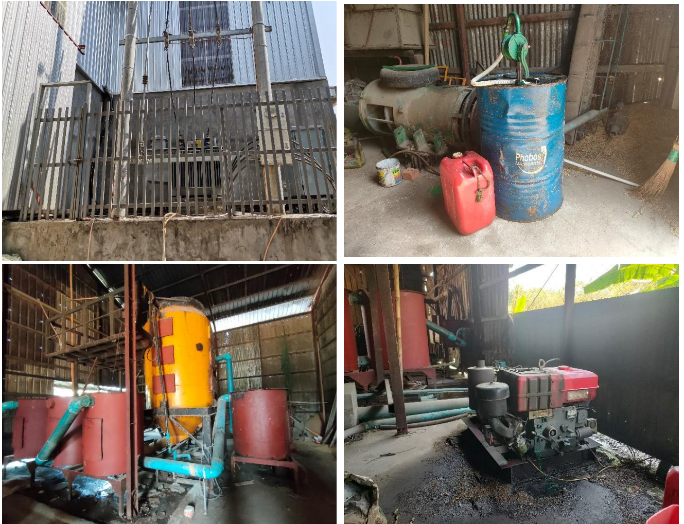
Figure 1-9 Electricity facilities at the Proposed Project
