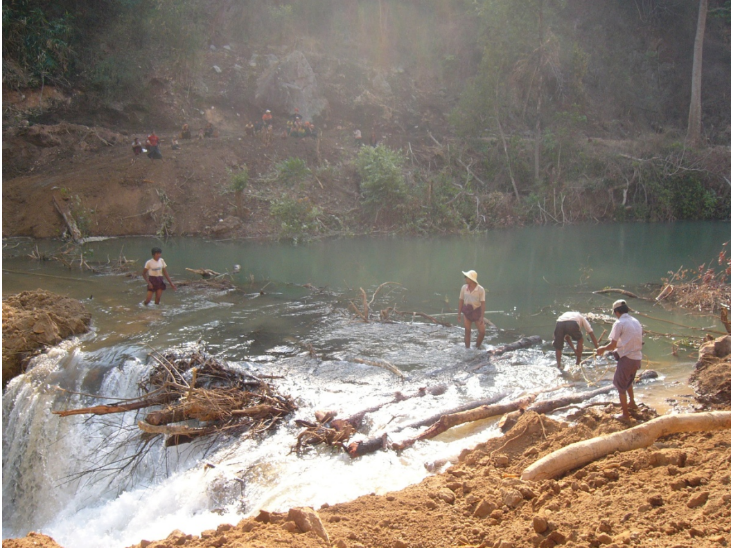
Photo ( 3 ) Under construction of BH5 drill pad at Balu chaung stream section
