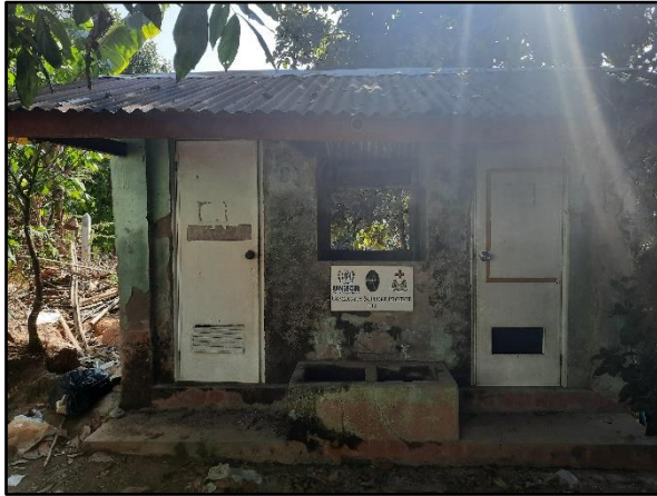
Septic Tanks at School (Ma Sa Village)
