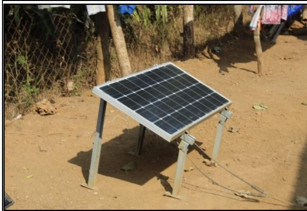
Solar Panel in Yar Do Village
