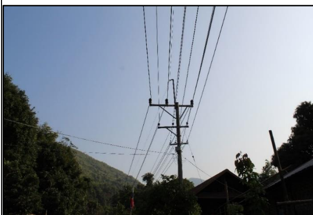
Existing Electricity lines in Kaw Bat Chan Village
