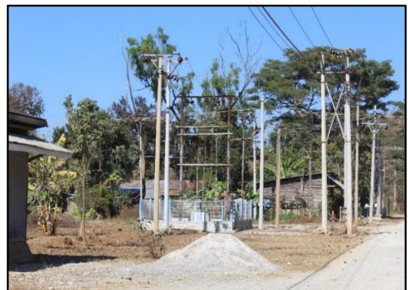
Electricity Infrastructure at Law Pi Ta Village
