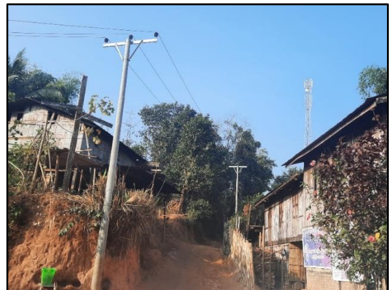
Existing Electricity Lines in Kyay Min Village
