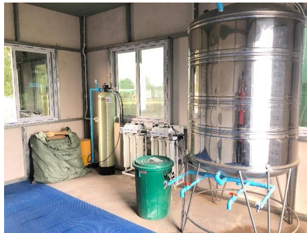
Figure 7. 6 Drinking Water Purification System
