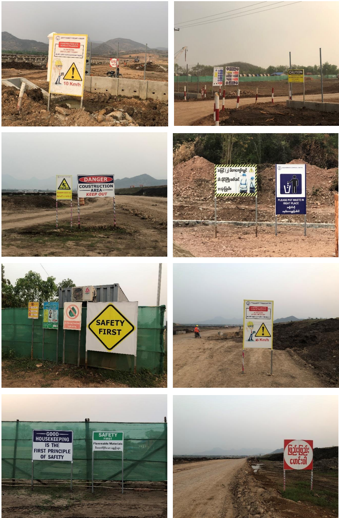
Figure 7. 4 Tagged Safety Signages in the Project
