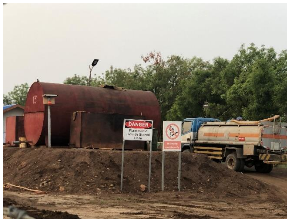
Figure 7. 3 Leak-proof Fuel Container in the Project
