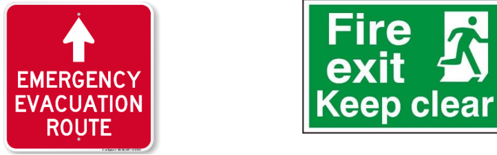
Figure 7.1 Firefighting Equipment and Singage
