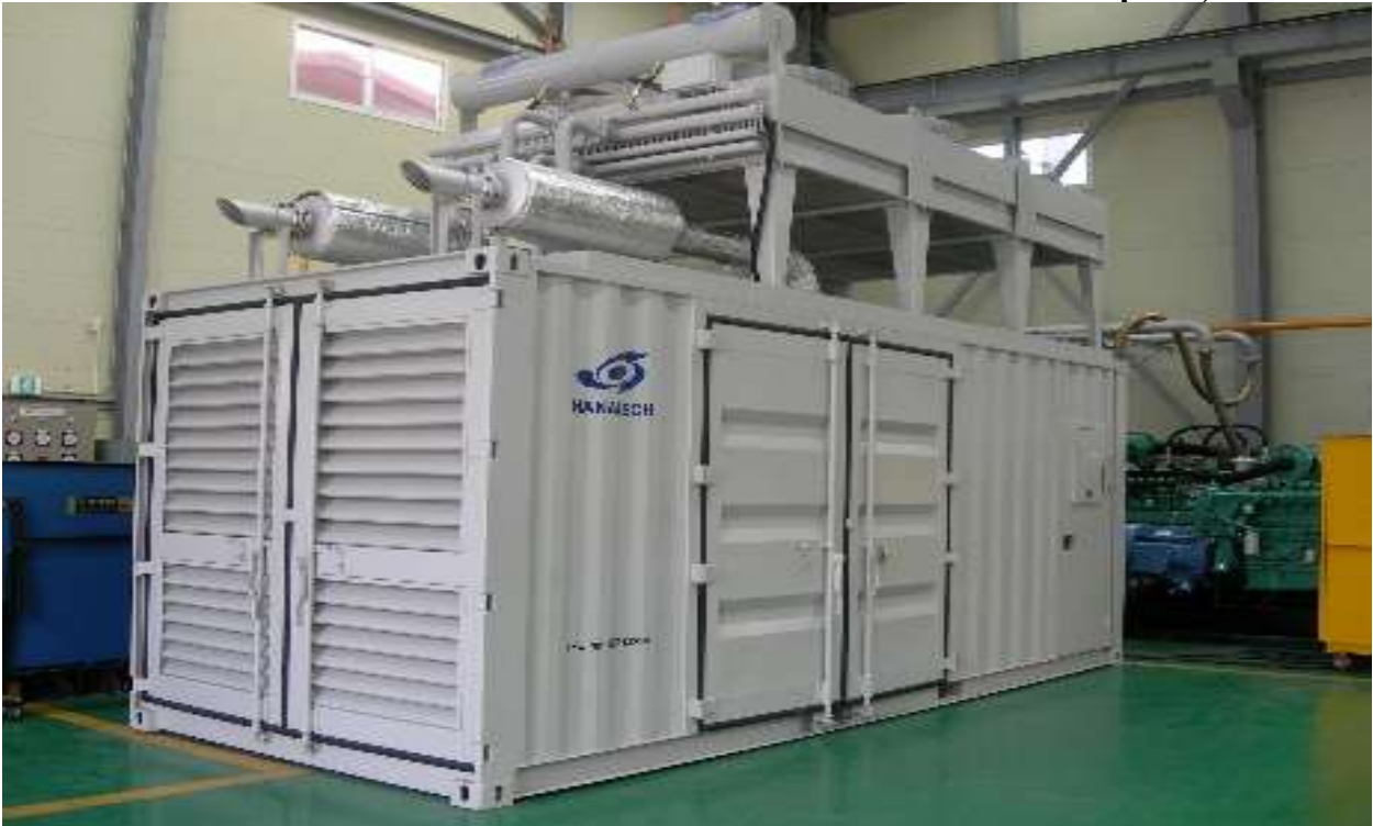
Figure 4.20: Sound and weather proof type generator
