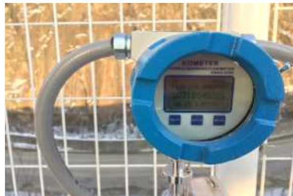
Gas Flow Meter
