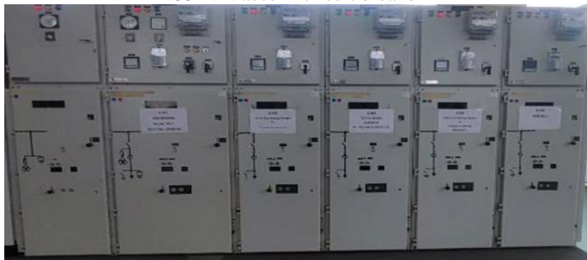
12 kV Vacuum-circuit breaker Switchgear
