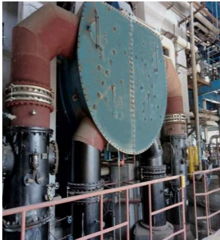
Figure – 25: Turbine condenser
