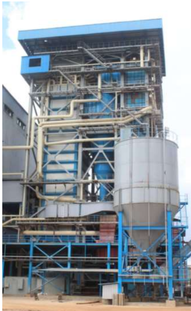
Figure – 10: Steam boiler (240 Tons)
