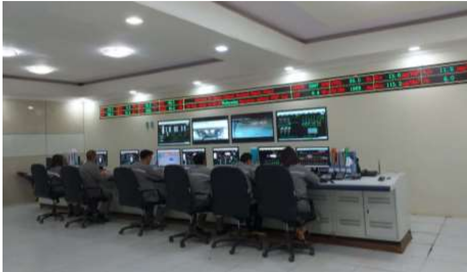
Figure – 43: Central Control Room (C.C.R)
