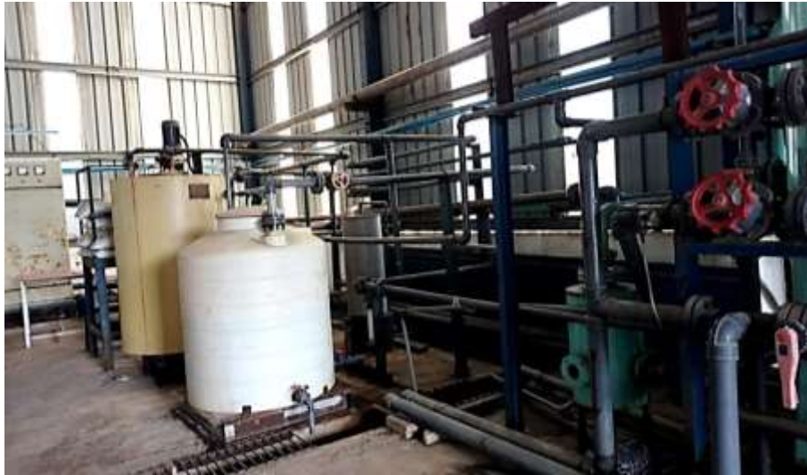
Figure – 52: Regeneration System (Feed Tank)
