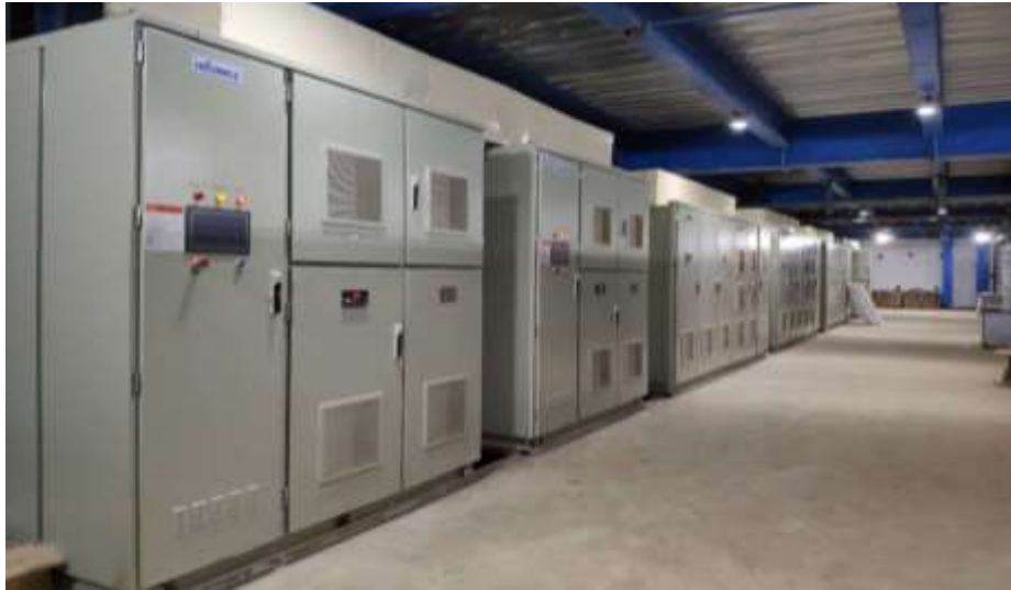
Figure – 37: Converter control panel
