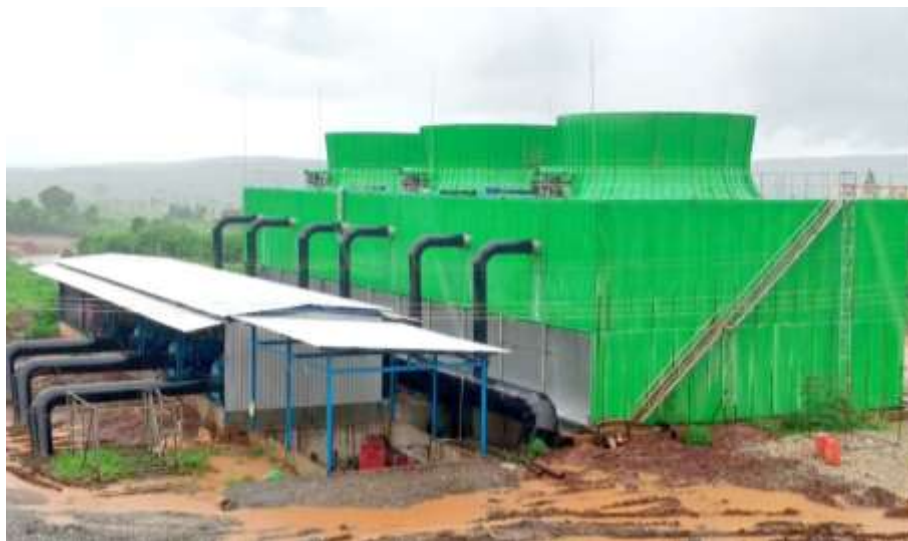
Figure – 71: Cooling Tower
