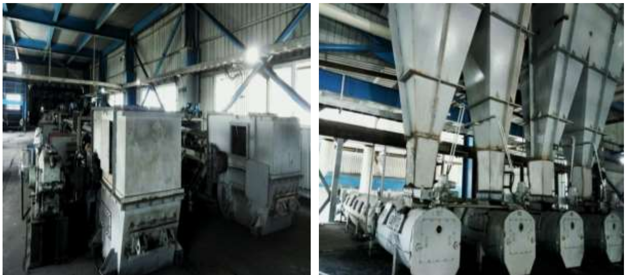
Figure – 15: Coal hopper
