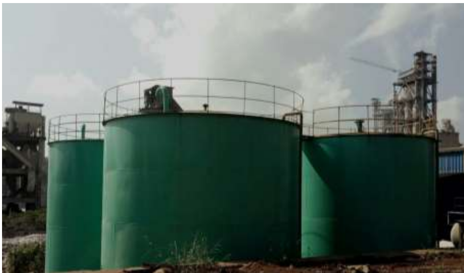
Figure – 54: R.O purified water tank
