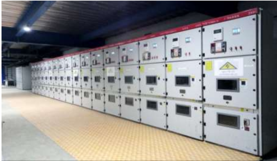
Figure – 40: Low voltage panel
