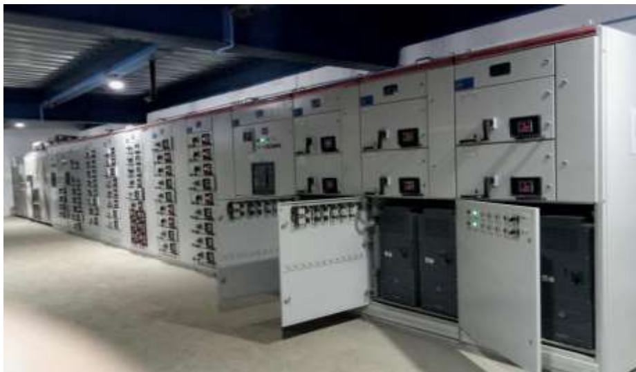
Figure – 39: High voltage panel
