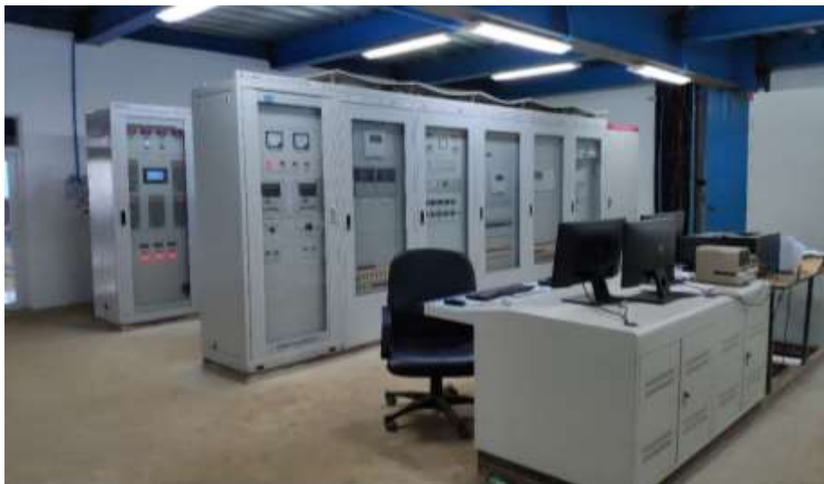
Figure – 42: Distribution control system (DCS)
