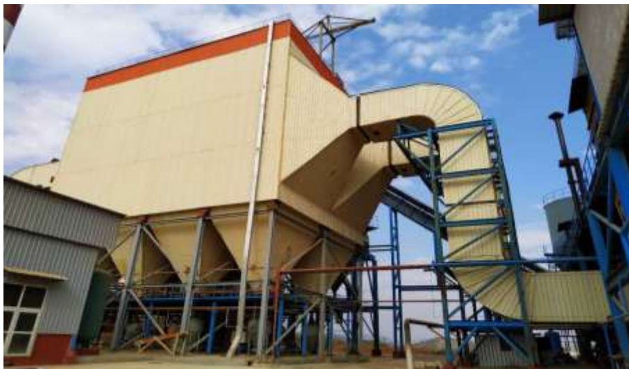
Figure – 29: EP Dust Collector
