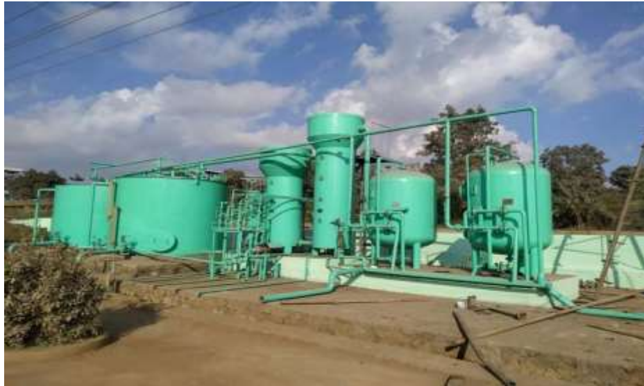
Figure – 73: Waste water/used water treatment plant
