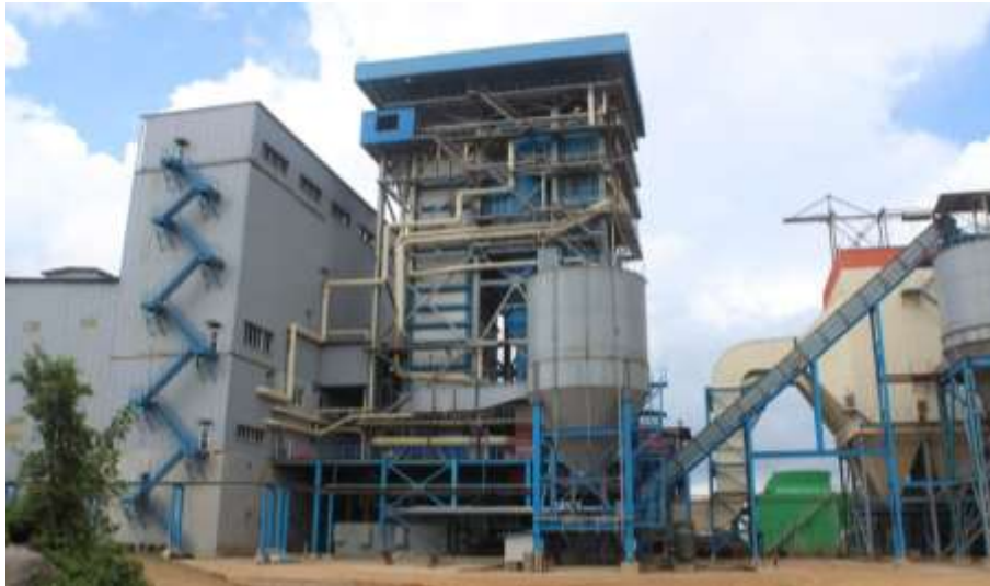
Figure – 11: Boiler & Turbine
