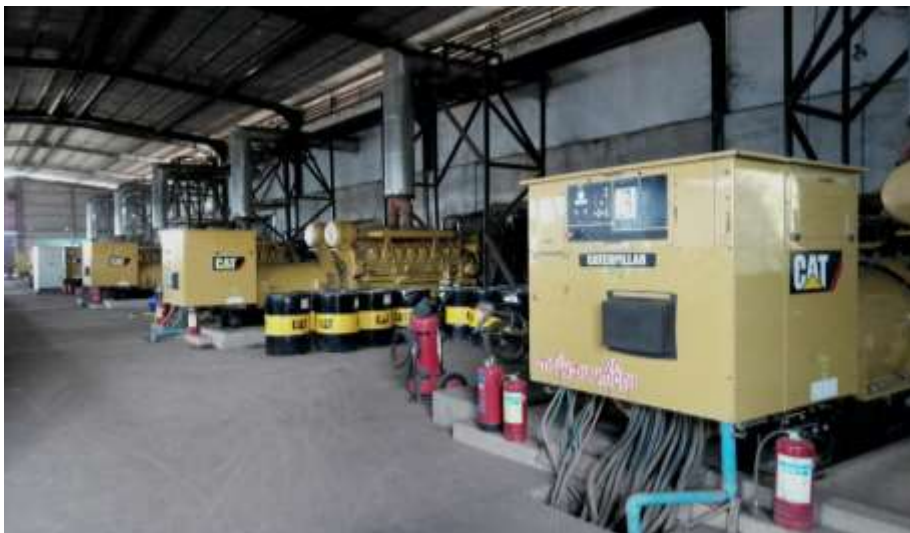
Figure – 21: Backup generators
