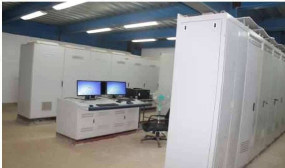
Figure – 41: Distribution control system (DCS)
