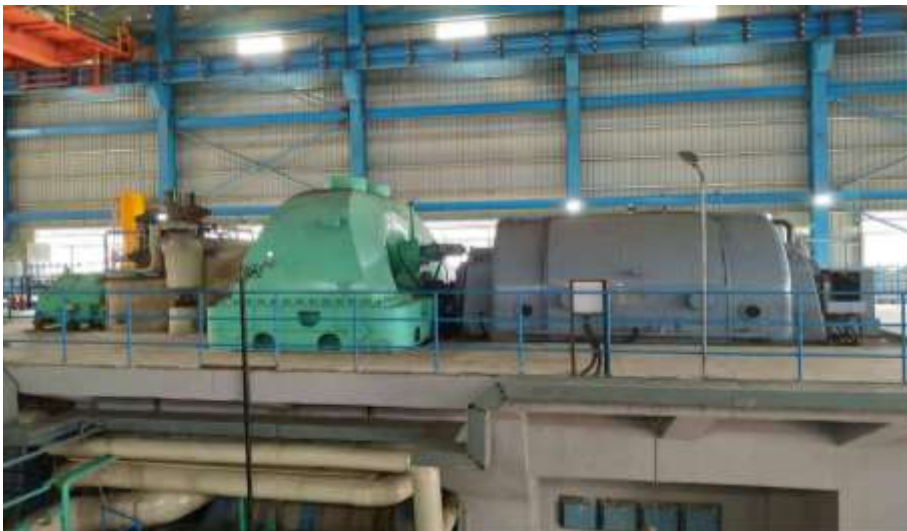
Figure – 20: 60 MW Steam turbine generators
