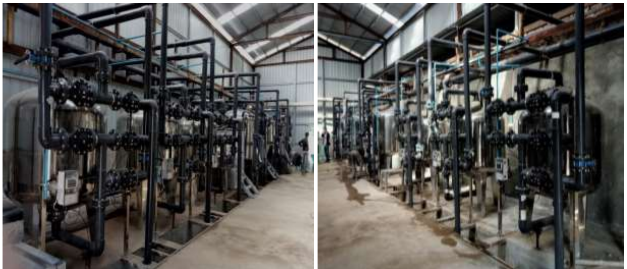
Figure – 57: Mechanical filters and Zeolite softeners
