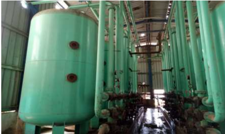
Figure – 55: Water softener
