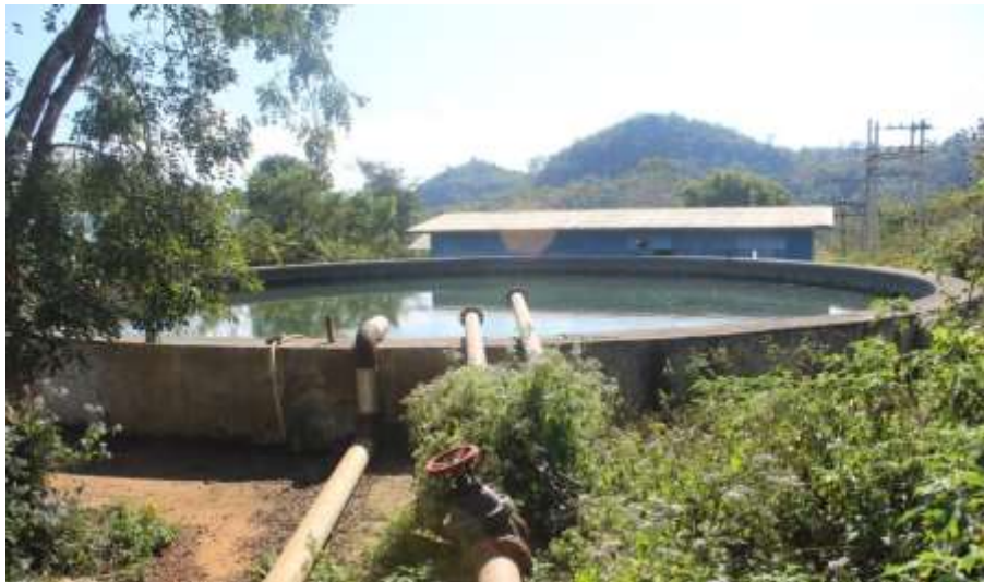
Figure – 50: 100,000 gallons water tank
