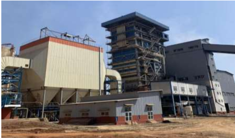
Figure – 28: Boiler, Turbine, EP Dust collector and Air compressor
