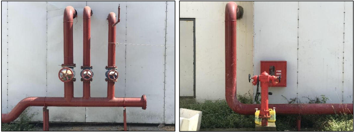
Figure 7-3: Fire Protection Water Tank and Pipe Line
