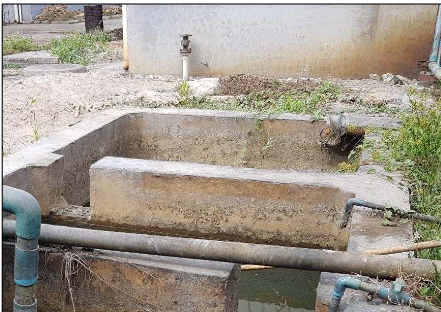
Figure 4-12: Boiler Blow Down Water Tank
