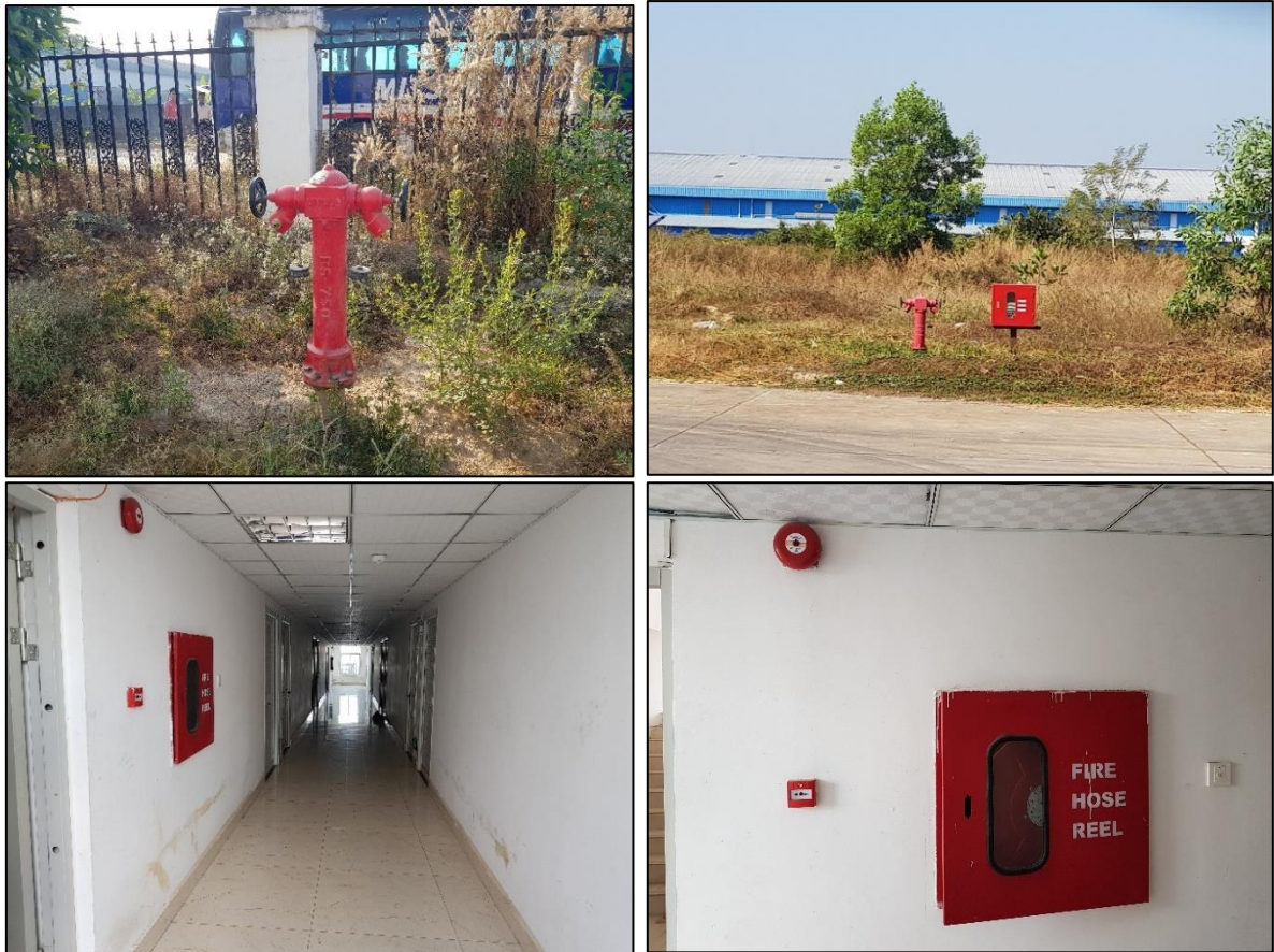
Figure 7-2: Fire Safety Equipment and Accessories
