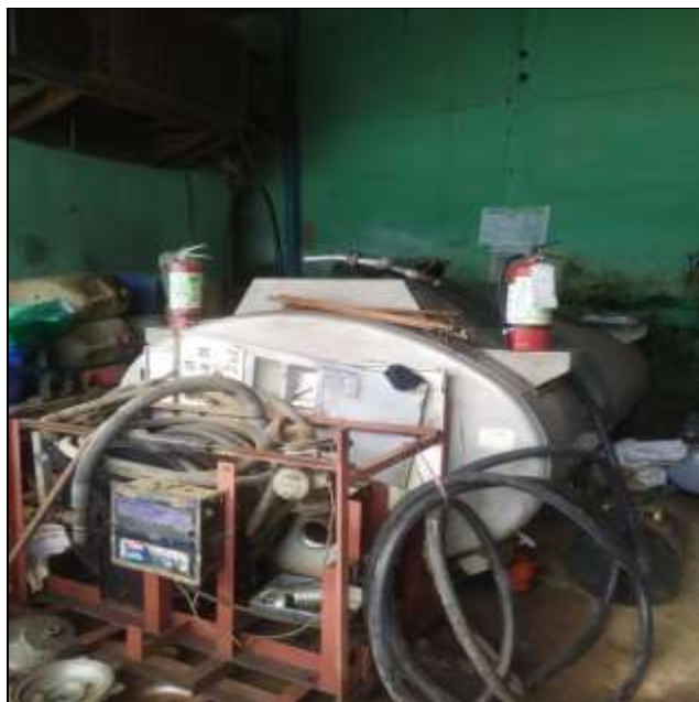
Figure 4. 13 Diesel Filling flowmeter
