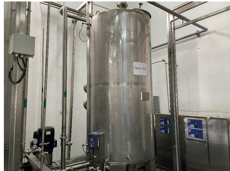
Figure 3-13 Water purification photo in September 6, 2022
