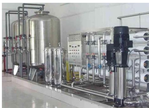
Water Treatment System
