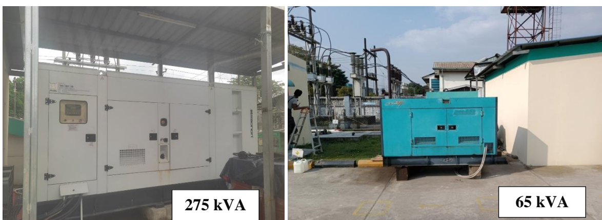
Figure 3.13 Photo of Diesel Generators (275 kVA) and (65 kVA) respectively
