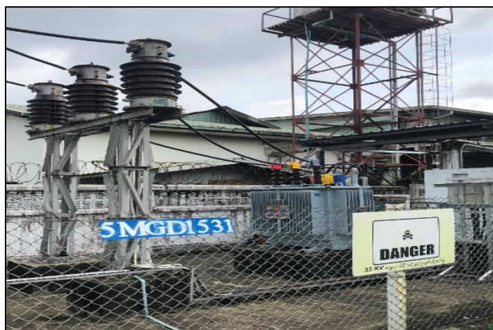
Figure 3.12 Photo of 315 kVA Transformer
