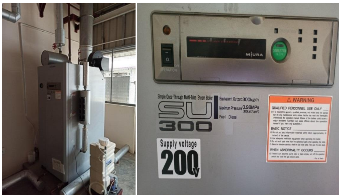
Figure 3.6 Photo of Diesel Boiler
