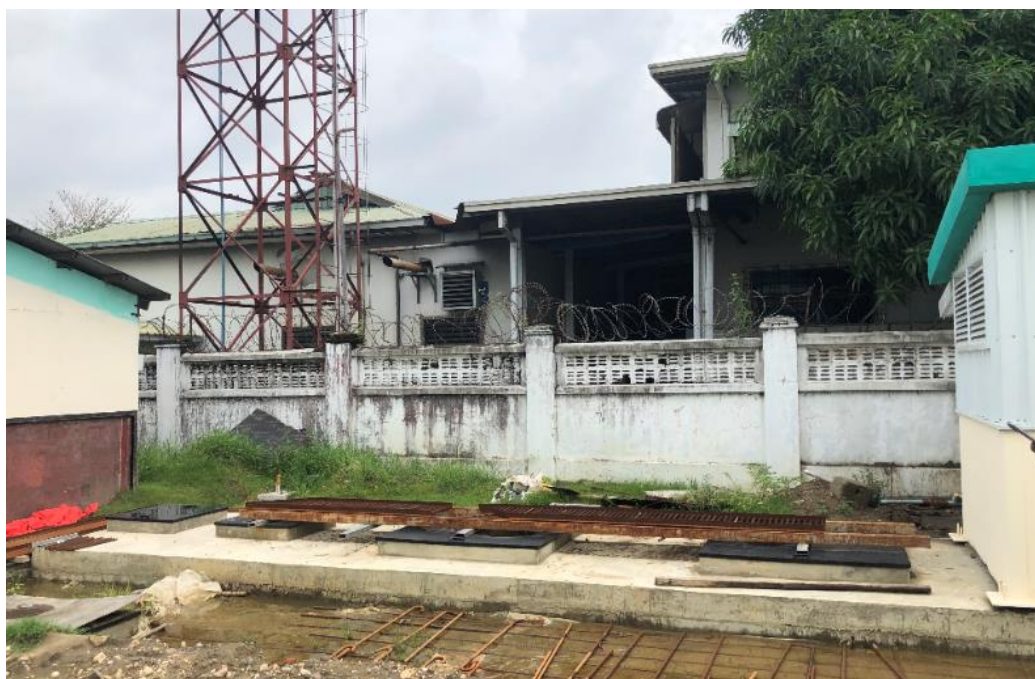
Figure 3.22 Photos of Installed WWTP
