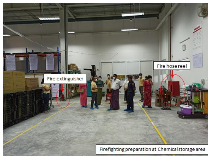
Figure 3.10 Photo of Firefighting Equipment Arrangement for Chemical Hazardous and Explosion
