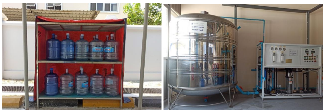
Figure 3.16 Photos of Drinking Water Supply
