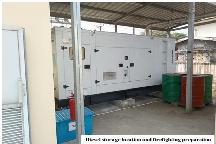
Figure 3.15 Photo of Main using Generator and Fuel Storage System
