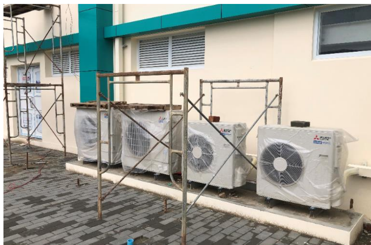
Figure 3.27 Photo of Air Conditioning System
