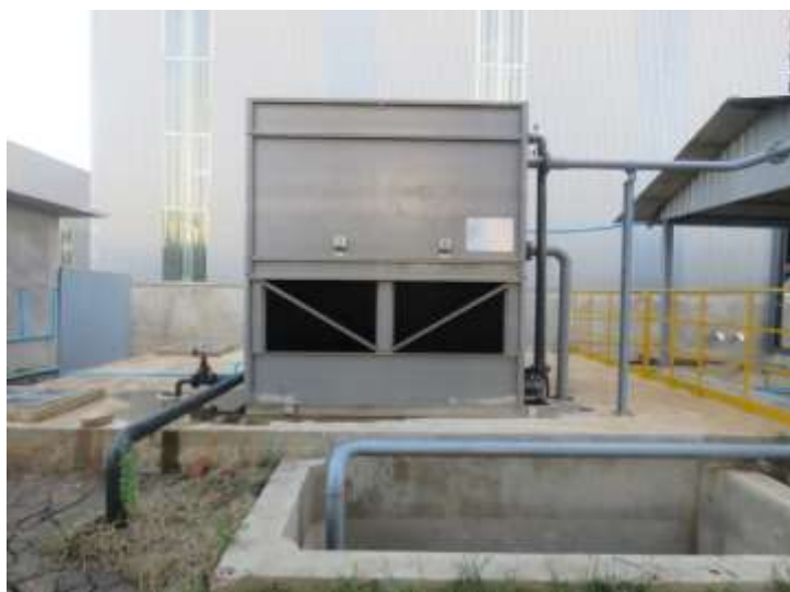
Figure-64: Cooling tower
