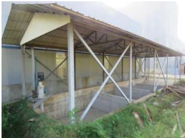
Figure-63: Four sedimentation tanks, waste water from waste water agitator tanks flows into this series of pond
