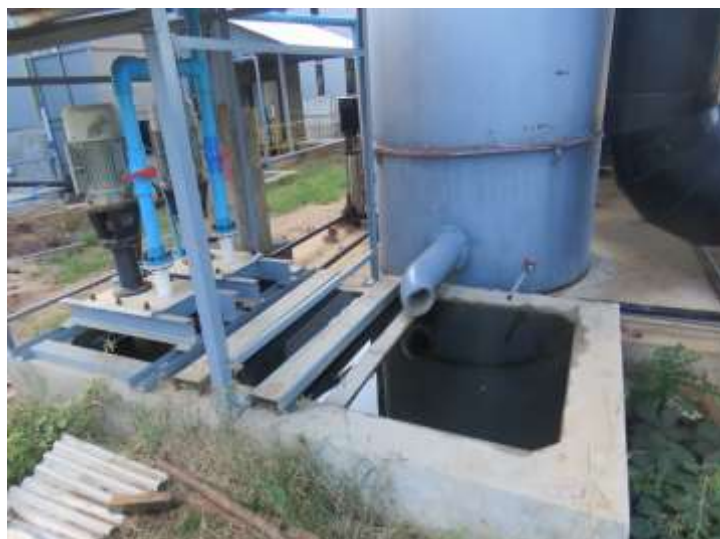
Figure-60: Ash pond (ash together with sprinkle water will flow down the pipe into the pond)
