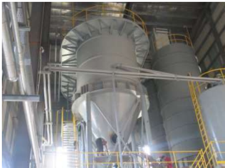
Figure-33: Clean water return tank
