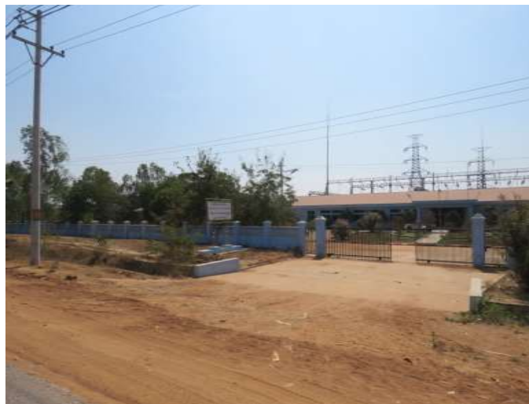
Figure-57: Bellin Sub-station
