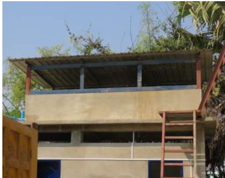
Figure-54: Elevated tank (for office and domestic uses)
