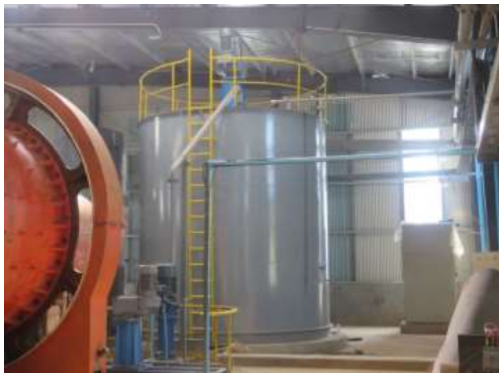
Figure-24: Slurry mixing tank
