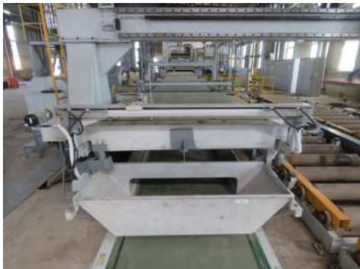
Figure-43: High pressure water cutter
