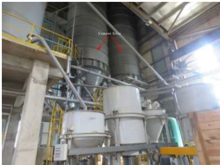
Figure-31: Cement silos
