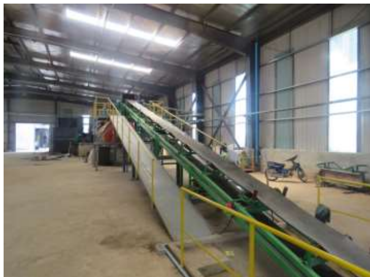
Figure-22: Conveyor line
