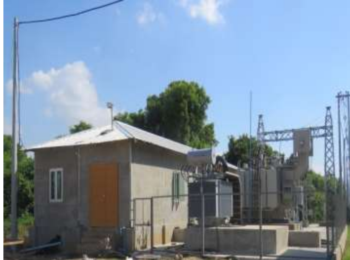
Figure-58: Control room and transformer station
