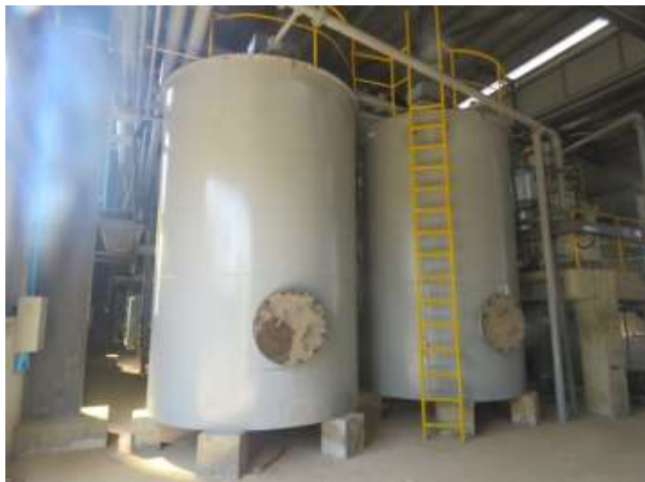
Figure-36: Cement and auxiliary materials silos
