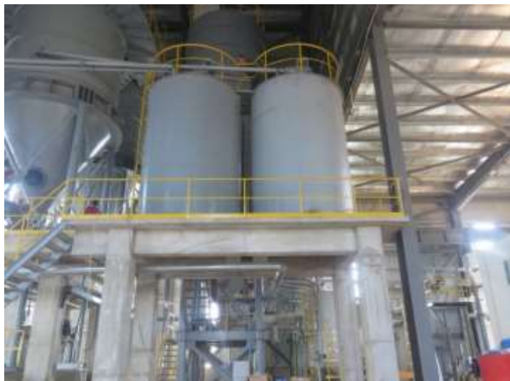
Figure-30: Pulp and sand tanks
