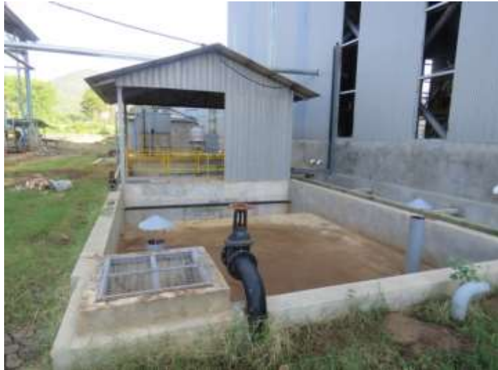
Figure-62: Waste water collection tank (used water/condense water from autoclaves flows into this pond)
