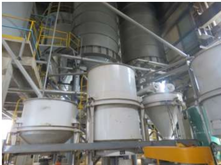
Figure-34: Sand, pulp and cement tanks (From left to right)
