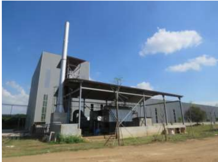
Figure-16: Boiler unit and stack
