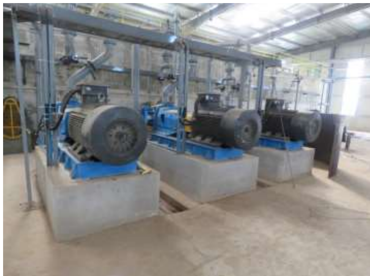
Figure-28: Pulp pumps
