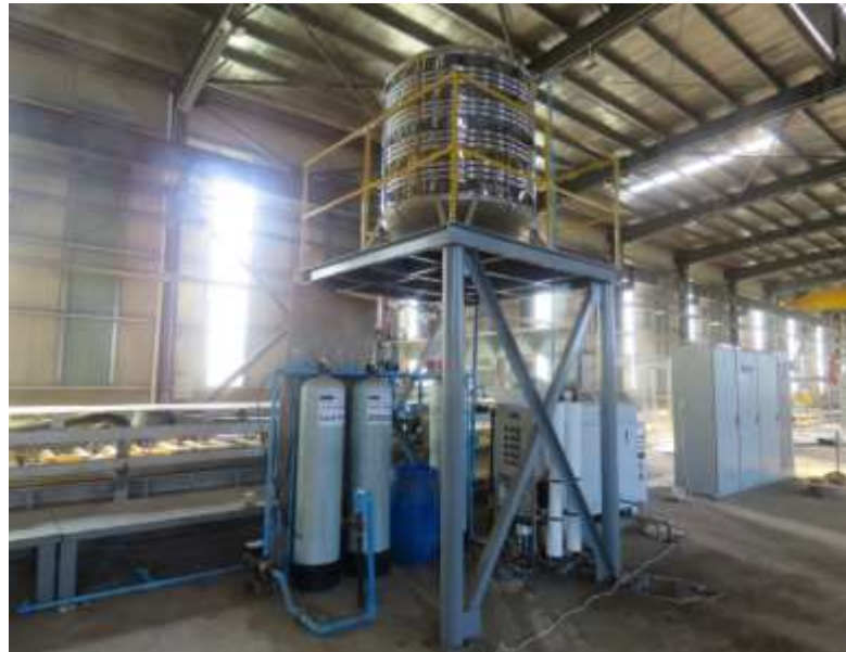
Figure-56: Water treatment unit
