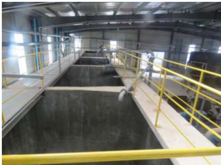
Figure-27: Slurry tanks
