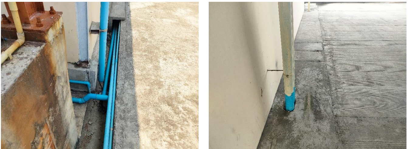
Figure 3-11 Drainage System of Factory
