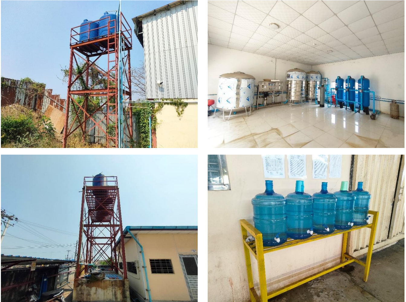
Figure 3-7 Water storage tank and drinking water supply
