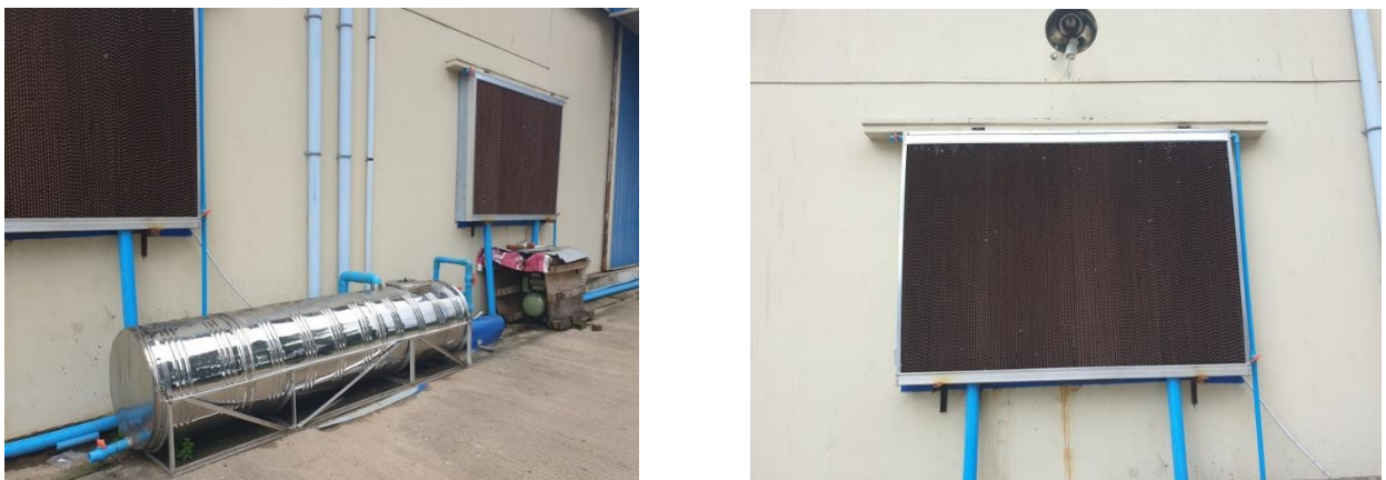
Figure 3-14 Ventilation System Photo
