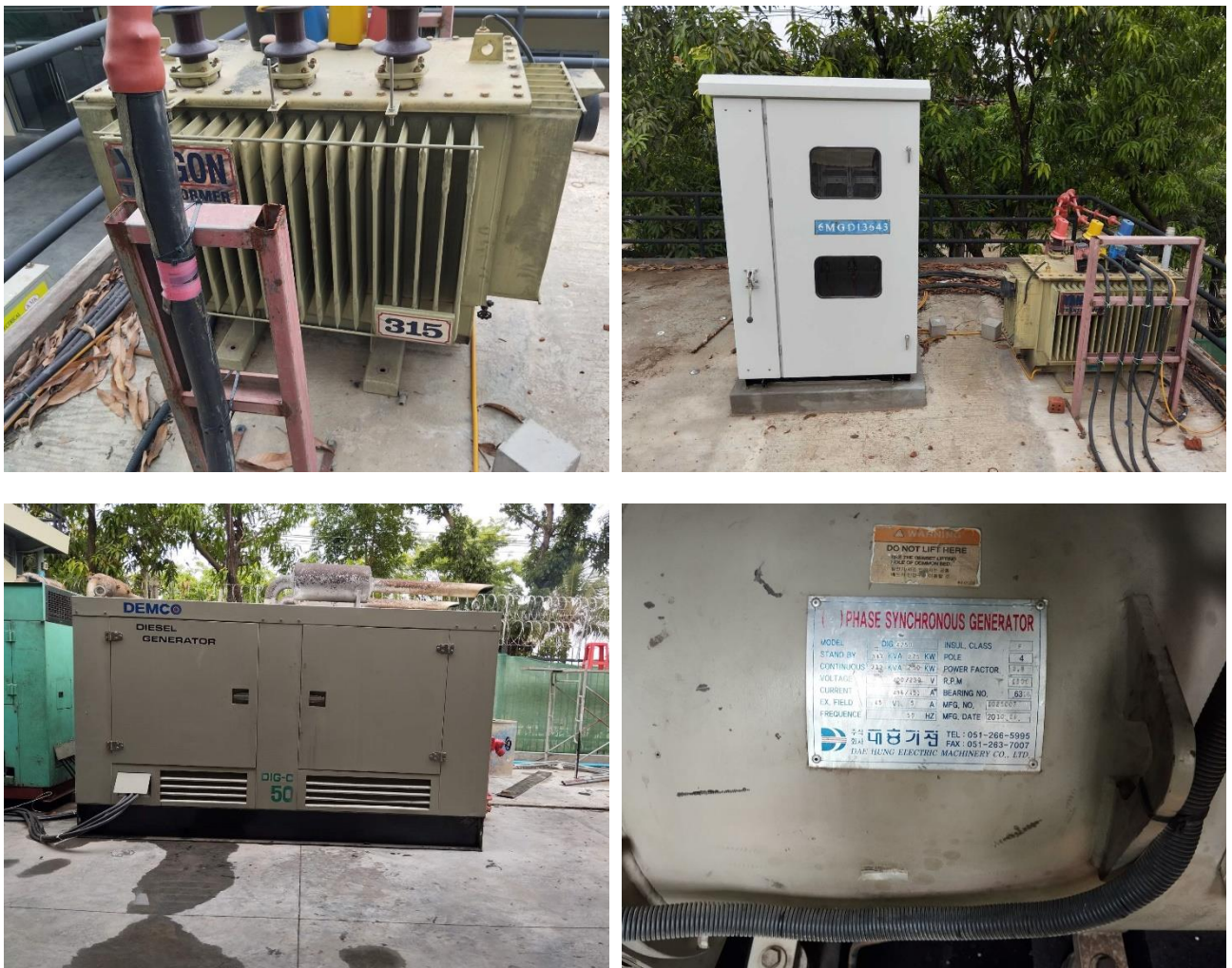
Figure 3-5: Transformer and Generator in the Factory
