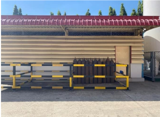
CO 2 & O 2 Gas Filling Station
