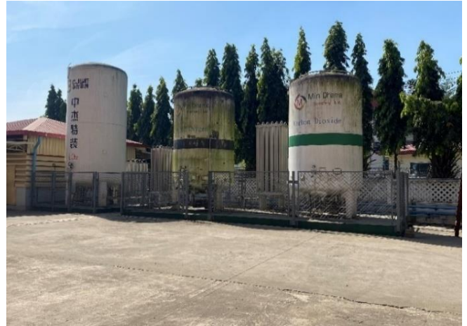
CO 2 & O 2 Gas Tanks
