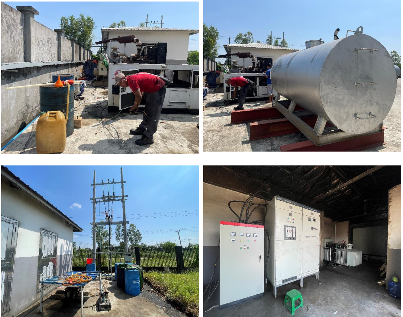
Figure 1-10 Generator Room and Fuel Storage Area
