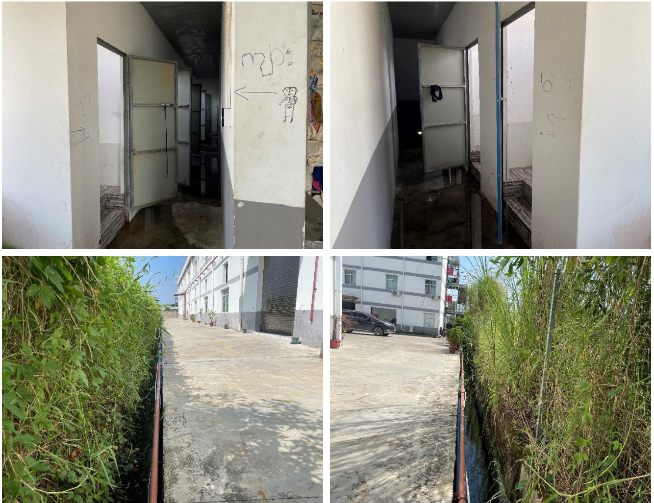
Figure 1-13 Toilets and Drainage photo
