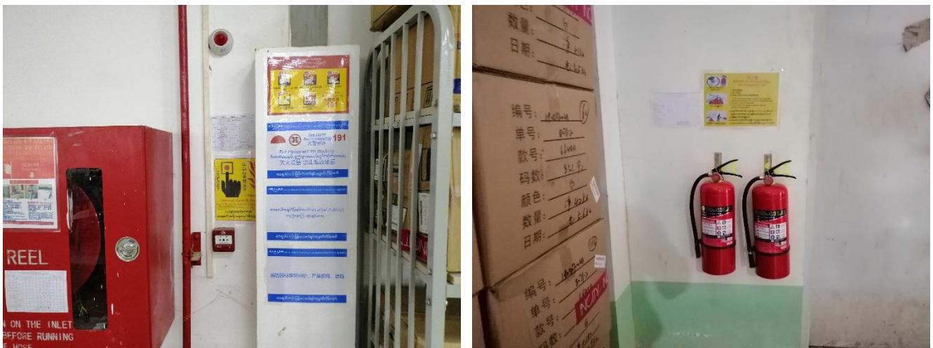
Figure 3-12 Firefighting Management Photo
