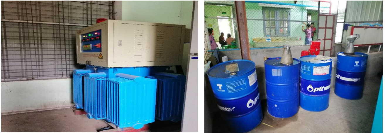
Figure 3-10 Electricity facility and fuel storage photo
