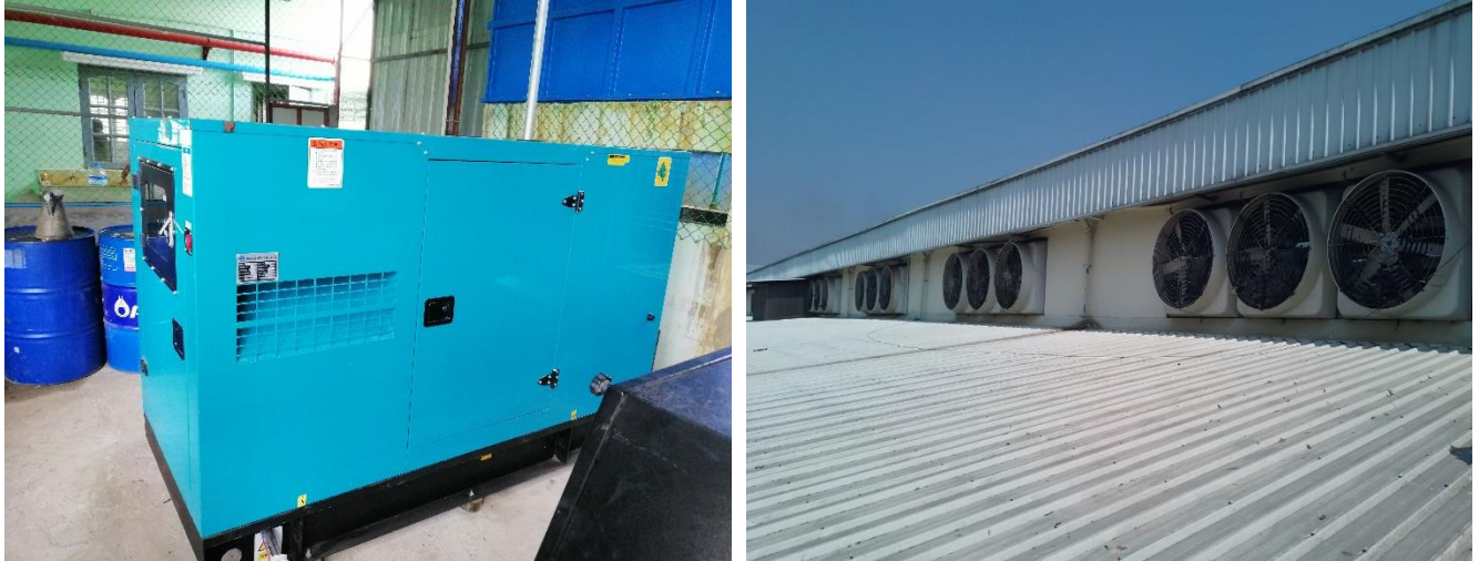
Figure 5-3 Moist fan and generator photo
