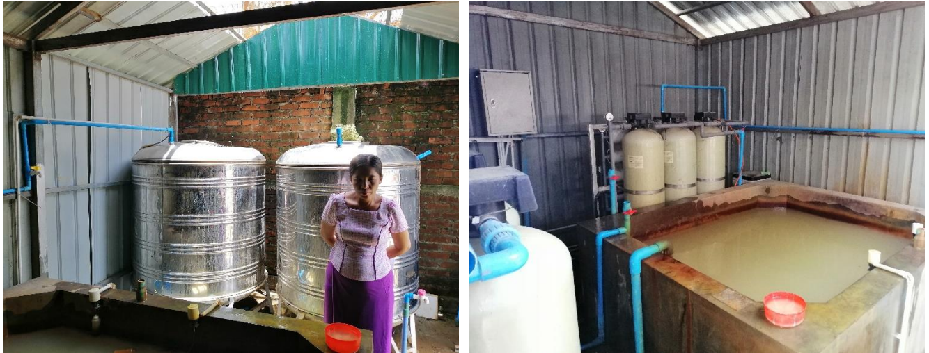
Figure 3-9 Overhead water storage tank and drinking water supply
