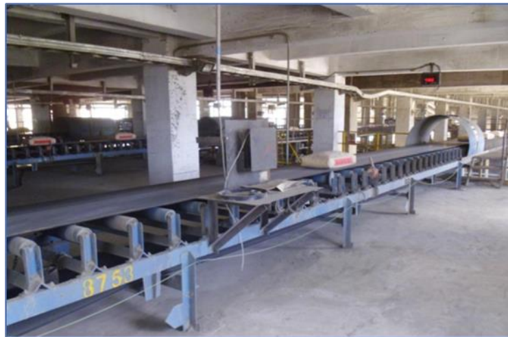
Figure 4.12 Packing Plant (Bag Conveying System)
