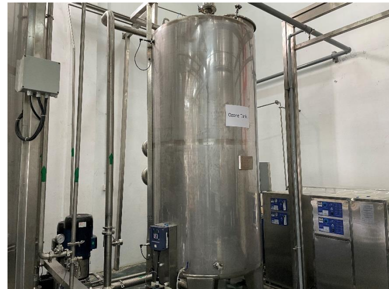
Figure 3-13 Water purification photo in September 6, 2022
