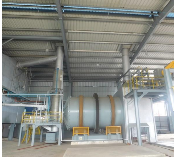
Figure 3.9-1: Rotary Furnace & Dust Line
