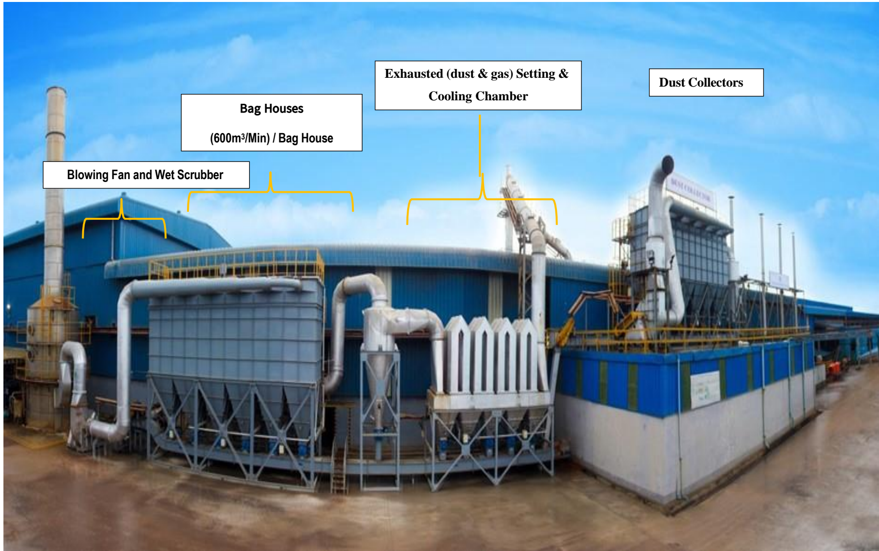
Figure 5.5.1-1: Air Emission Control Units in YMI Factory
