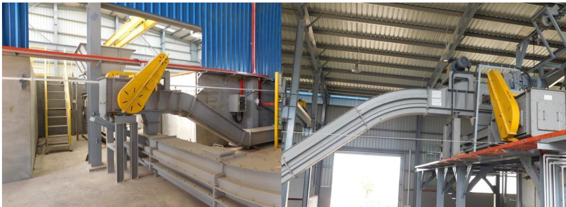
Figure 3.5-2: Chain Scrap Conveyor
