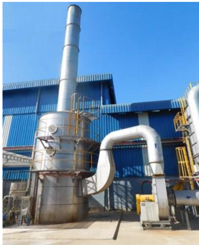
Figure 3.9-5: Blowing Fan and Wet Scrubber
