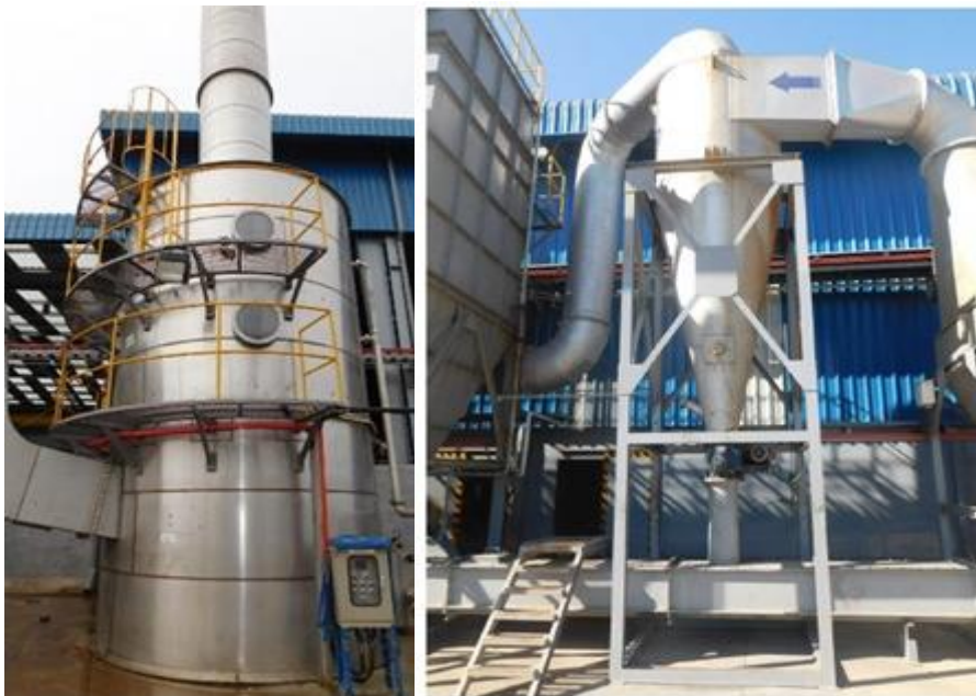
Figure 3.9-3: Exhausted (Dust & Gas) Setting & Cooling Chamber
