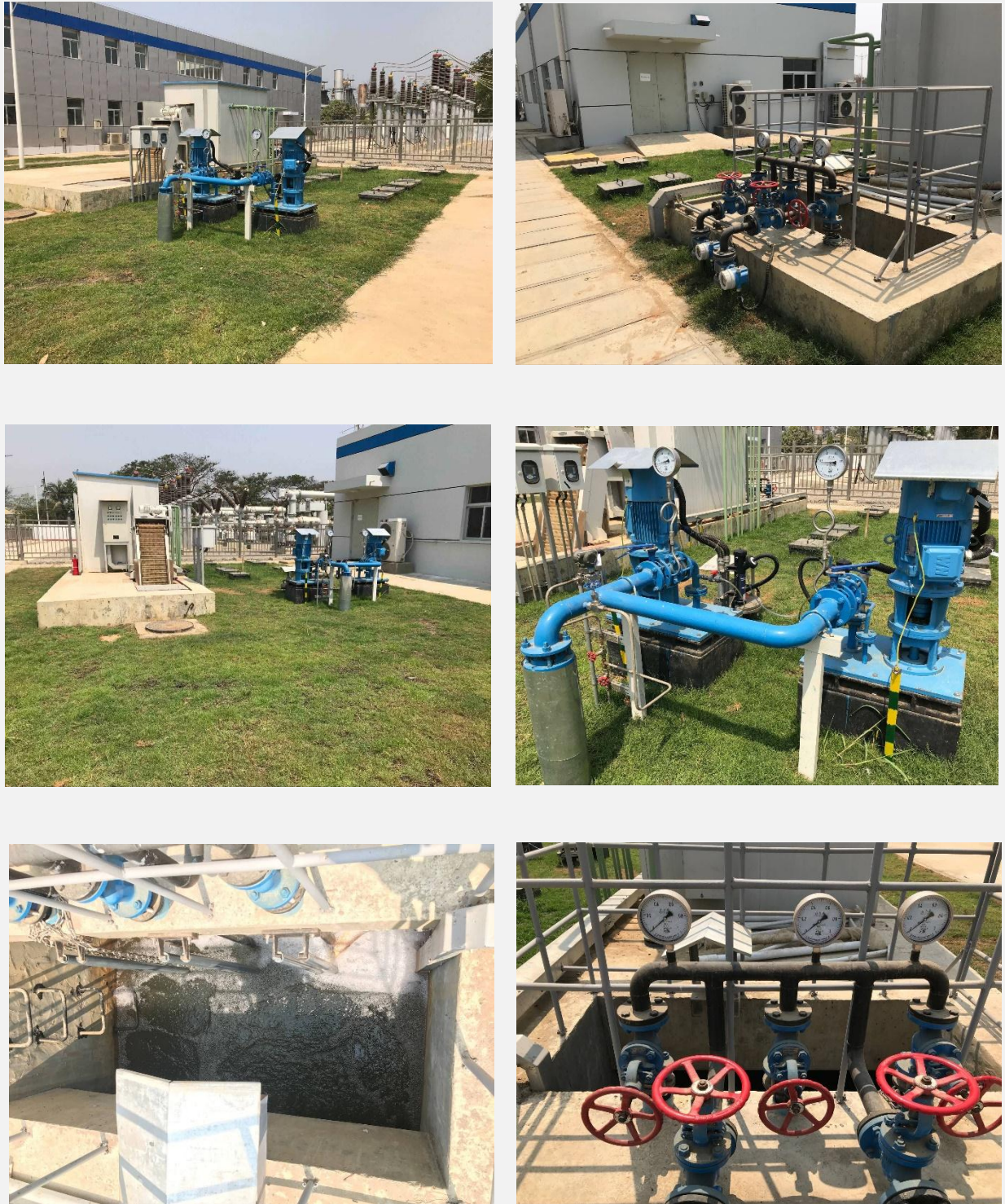
Figure 7.8-5 Sanitary Wastewater Treatment System
