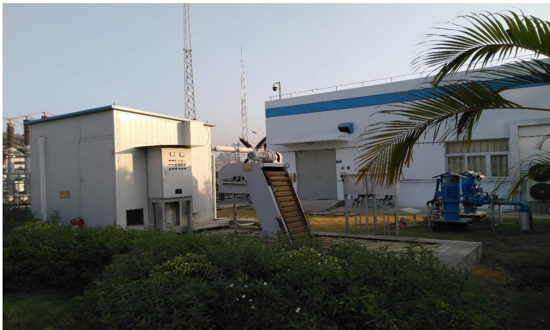
Figure 3.5-8: Sewage Water Treatment System
