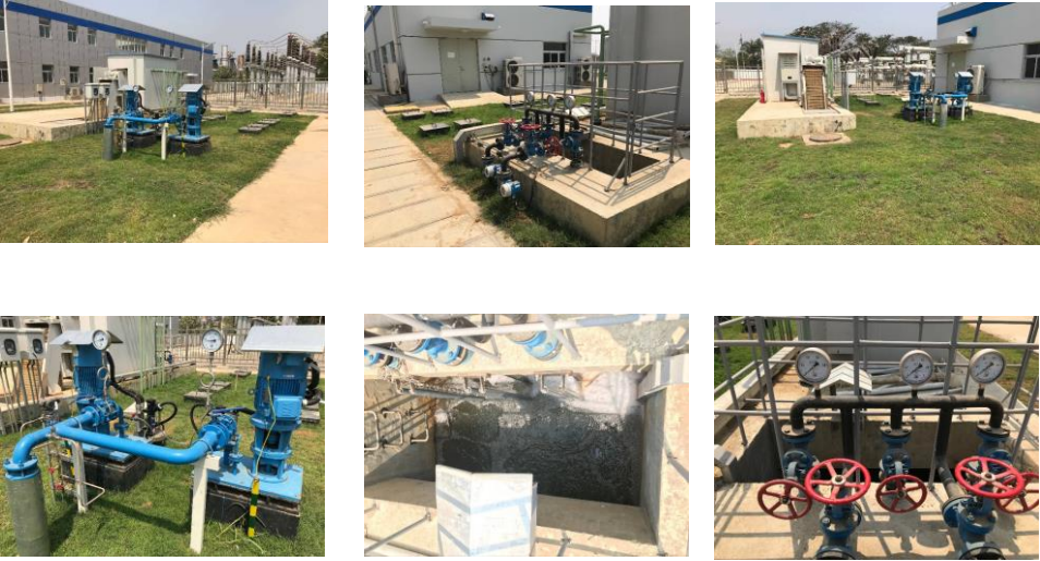
Pictures of Sanitary Waste Water Treatment System
