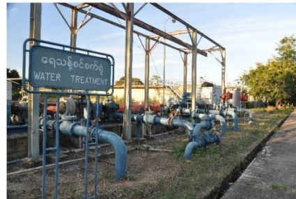
Water Treatment Factory
