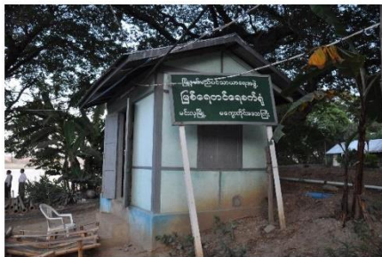
Minhla Water suction Pump
