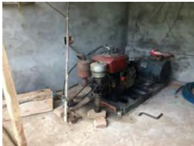
Photo Plate 5.51: Diesel Generator Set at Monastery in Yae Win Village
