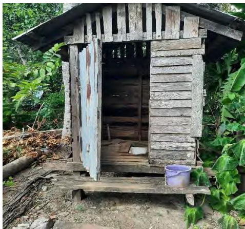
Photo Plate 5.48: Sanitation Facility at Myaung Shea
