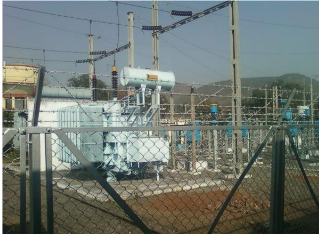
Figure - Future Railway Power Traction Substation
