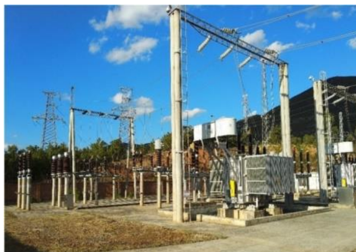
Fig. 4.20 - HV incoming side of traction substation
