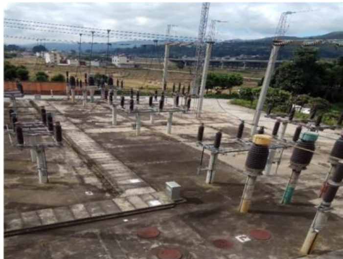
Fig. 4.19 - Vertical view of traction substation
