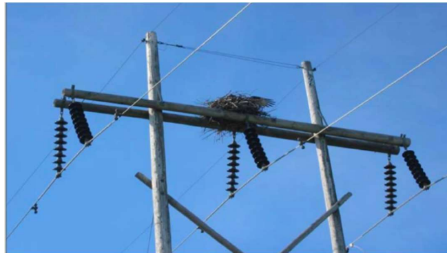
Hawks and eagles will occasionally use transmission structures as nesting sites
