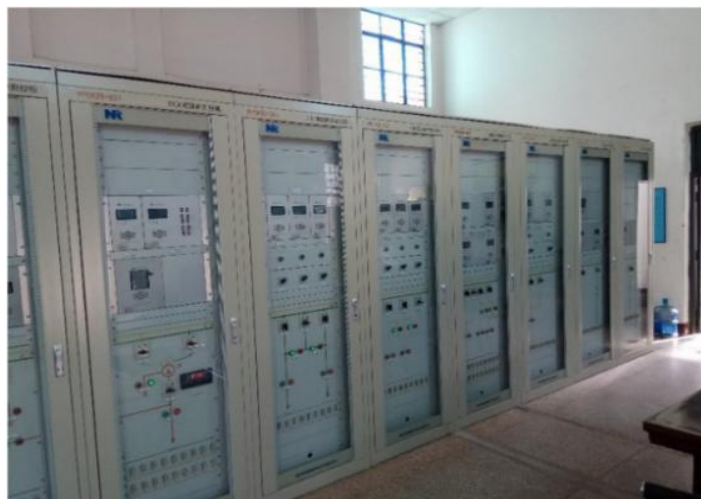
Fig. 4.21- Main control room of traction substation
