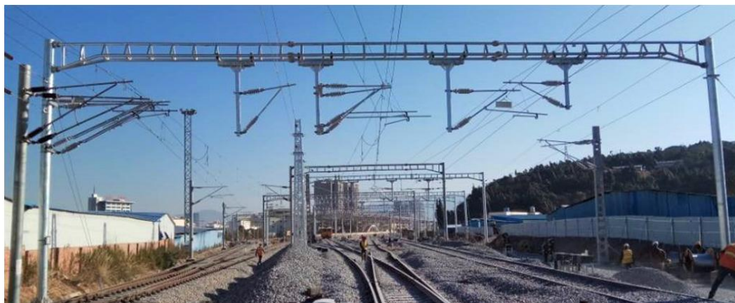
Figure. Hard cross-span of station
