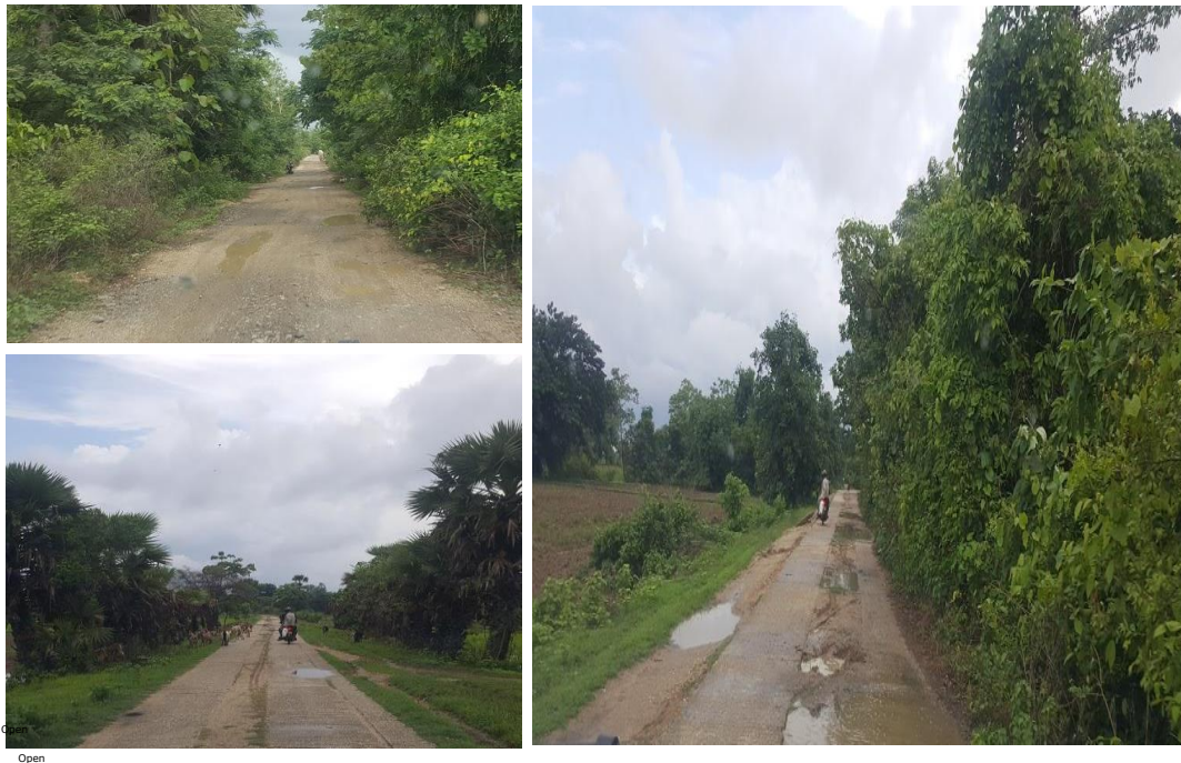
Figure 4-9: Present condition of MOGE Access Road
