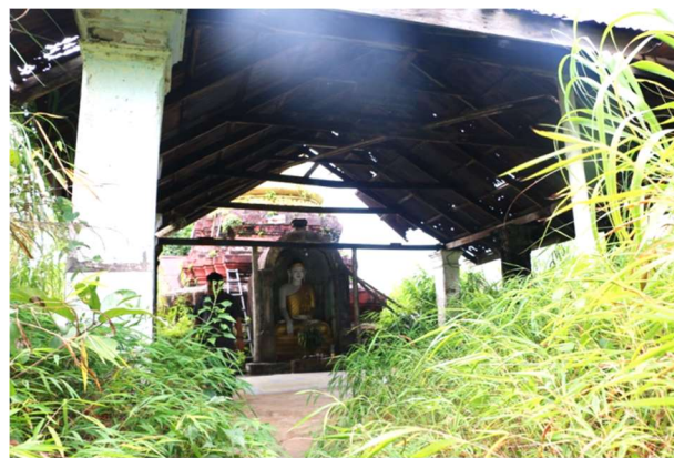
Figure - Pathat Pagoda Complex in the Lack of Maintenance
