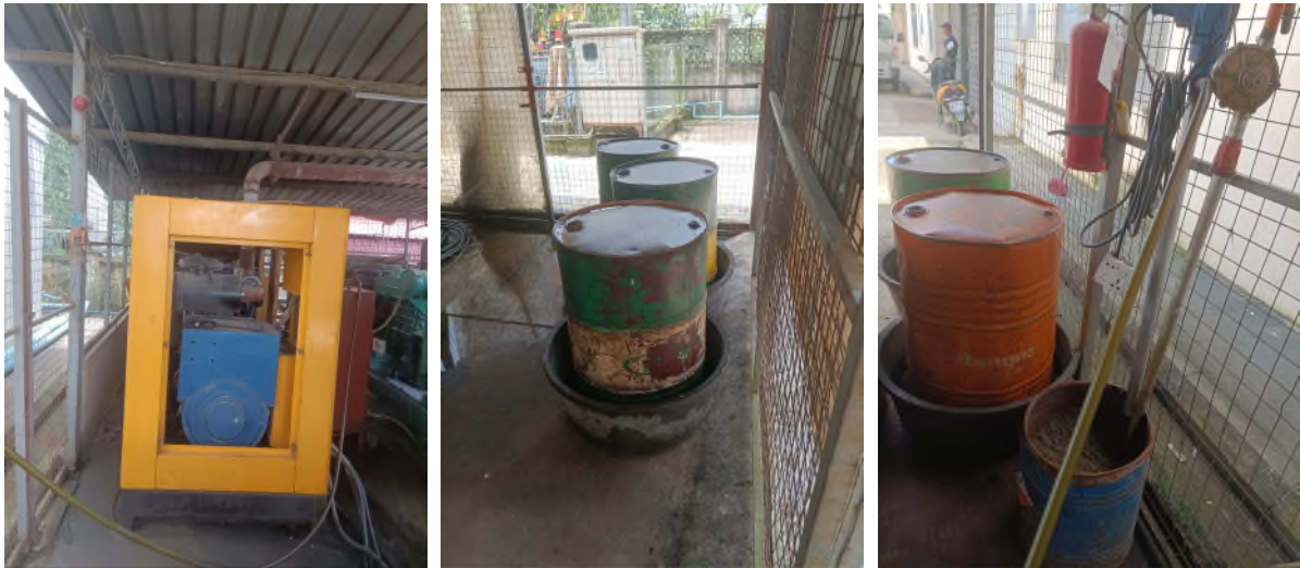
Figure 35: Diesel Fuel Storage
