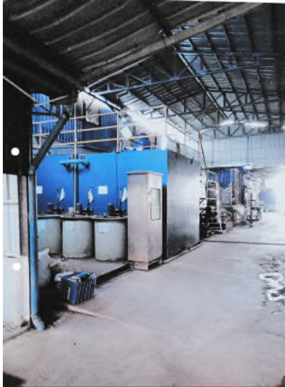
Dosing Equipment and layout
