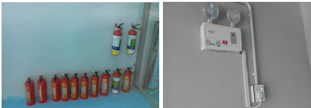
Figure 20: Fire extinguishers and alarms
