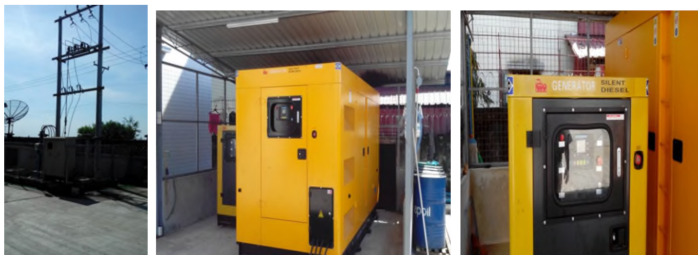
Figure 34: Transformer and Silent Type Diesel Generator
