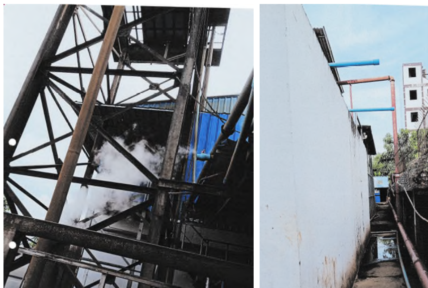
Figure 32: Overhead water tank, fire water tank and water line for firefighting
