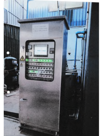
Wastewater treatment equipment
