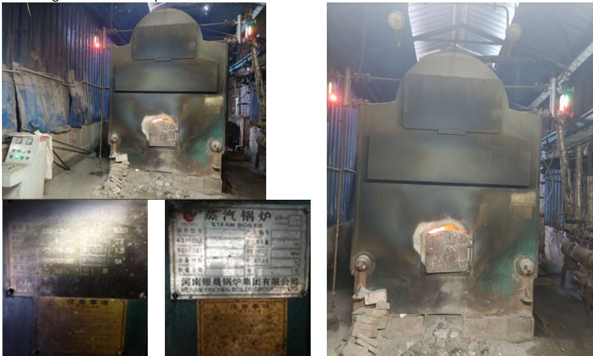
Figure 37: 1 MPa and 1.25 MPa Boilers at Myanmar Unique Garment Factory
