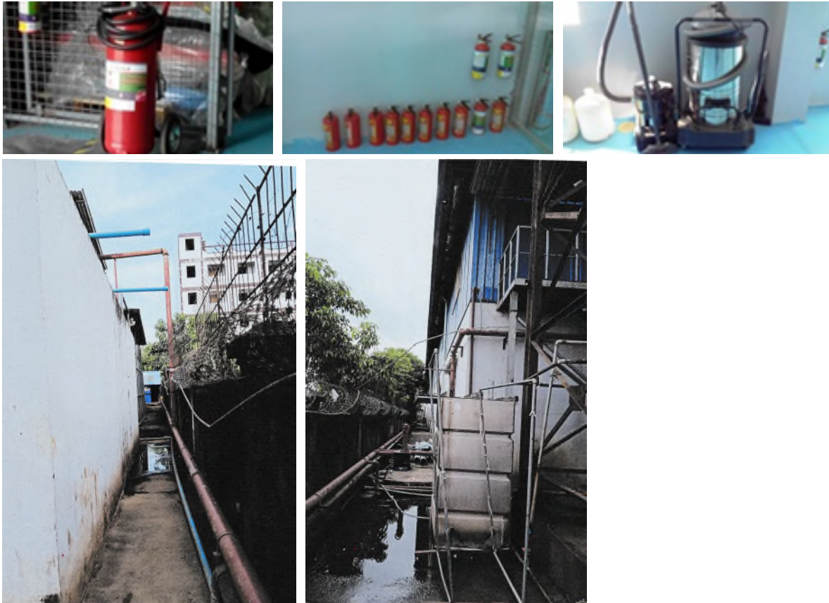
Figure 59: Firefighting Equipment and Fire water lines
