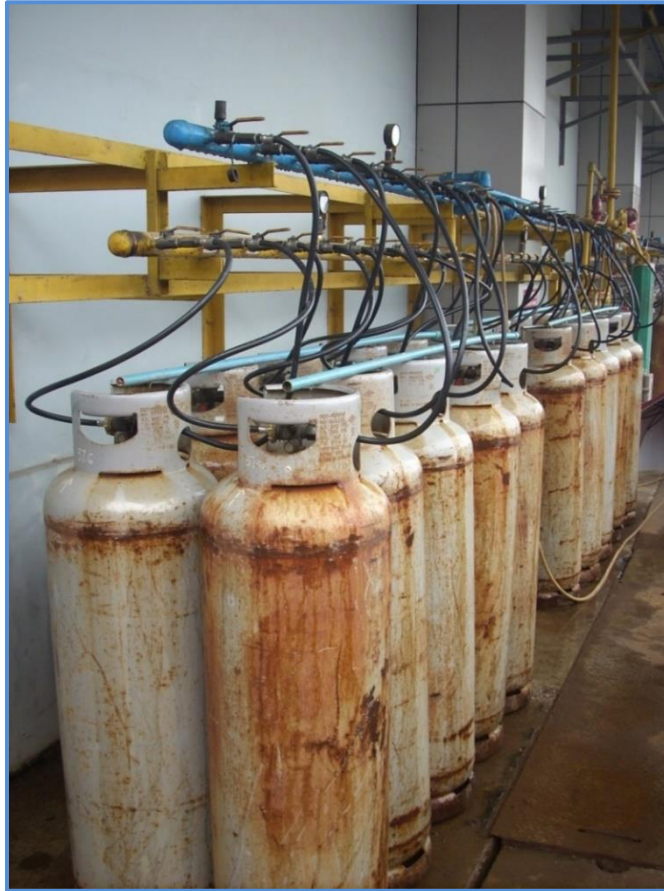
LPG Usage for oven at factory at Shwe Than Lwin
