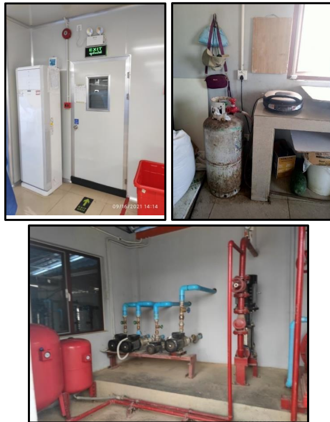
Figure 6-5 Installed Fire Extinguishers and Sprinkler, Water Hydrants, LPG and Fire Alarm System
