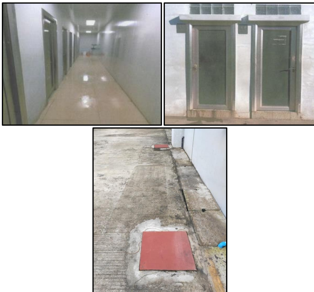
Figure 4-36 Toilets and Septic Tanks
