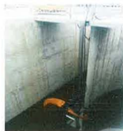
The Whole Equipment (Anaerobic Treatment)
