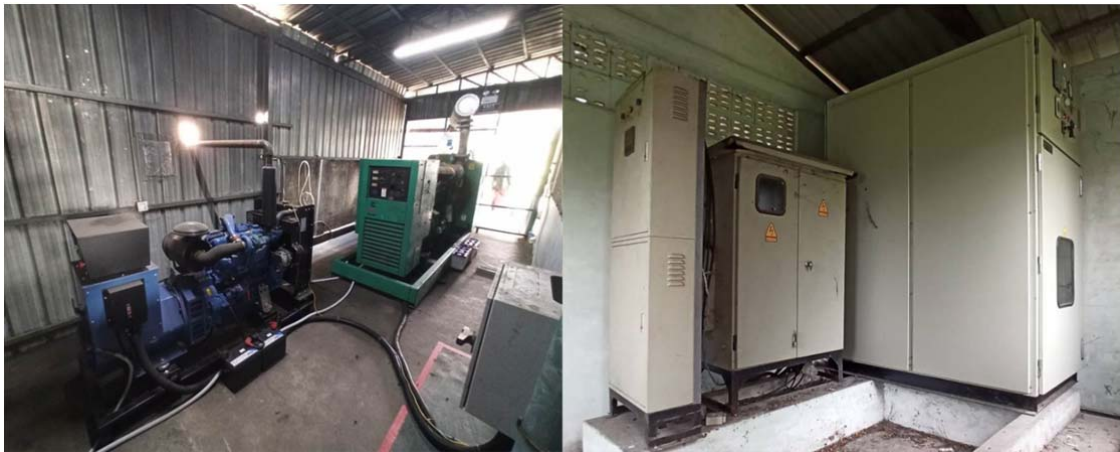
Figure 1-10 Electricity distribution room
