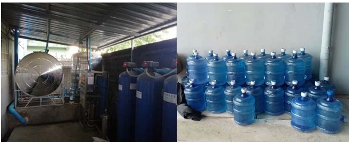
Figure 1-8 Water storage and filtration system
