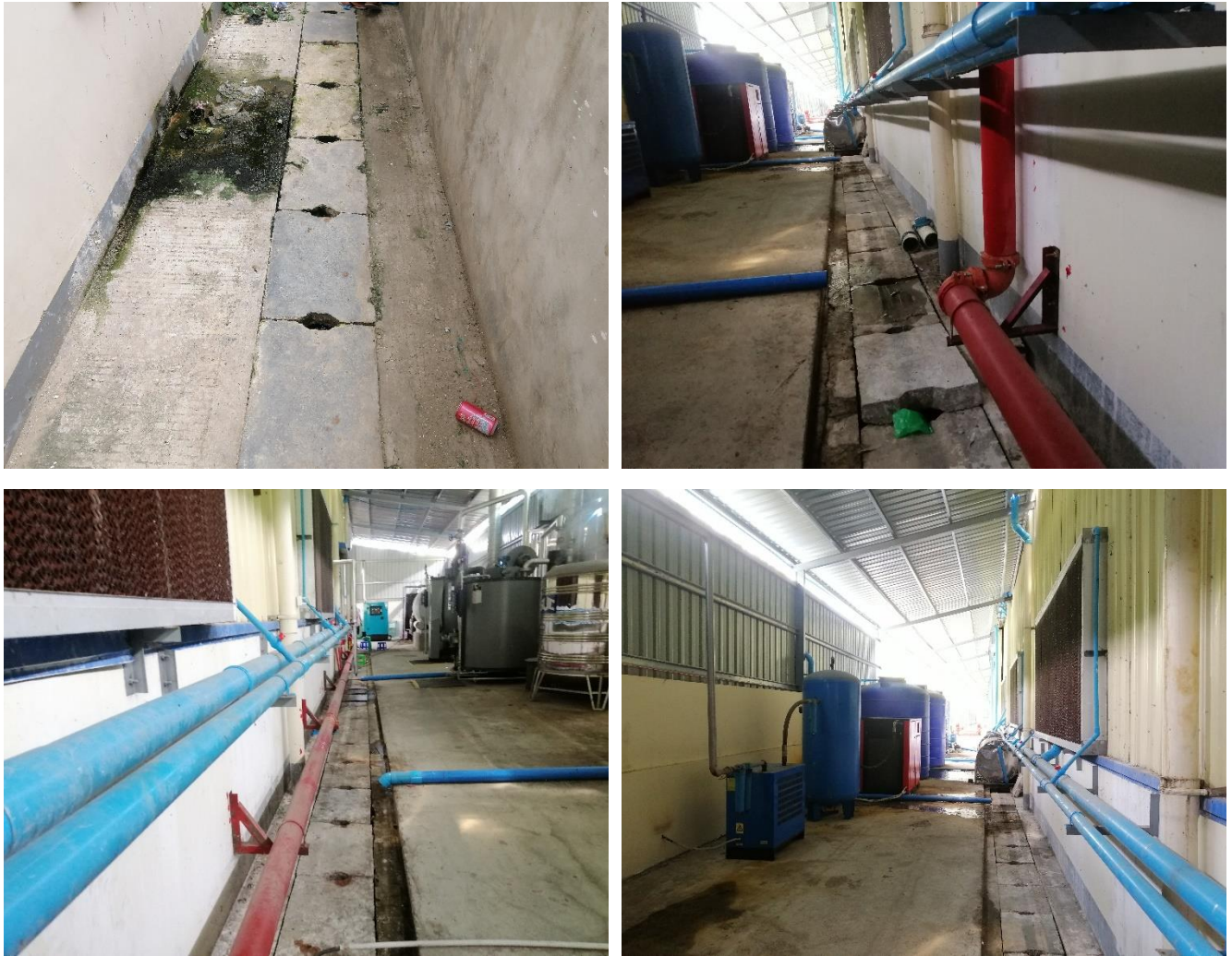
Figure 3-17 Water Drainage System
