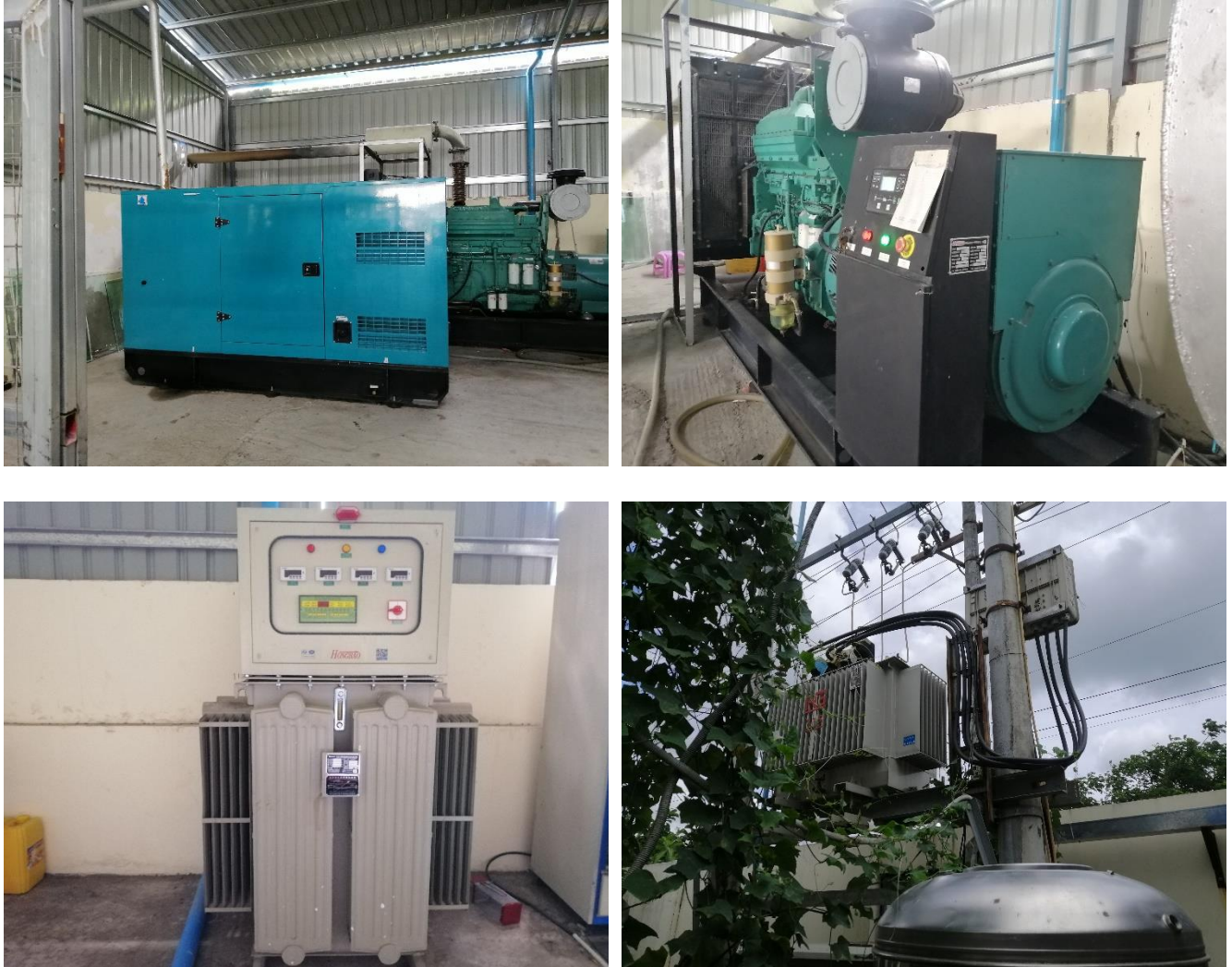
Figure 3-7 Electricity Facilities at Sunrise (Myanmar) Fashion Company Limited
