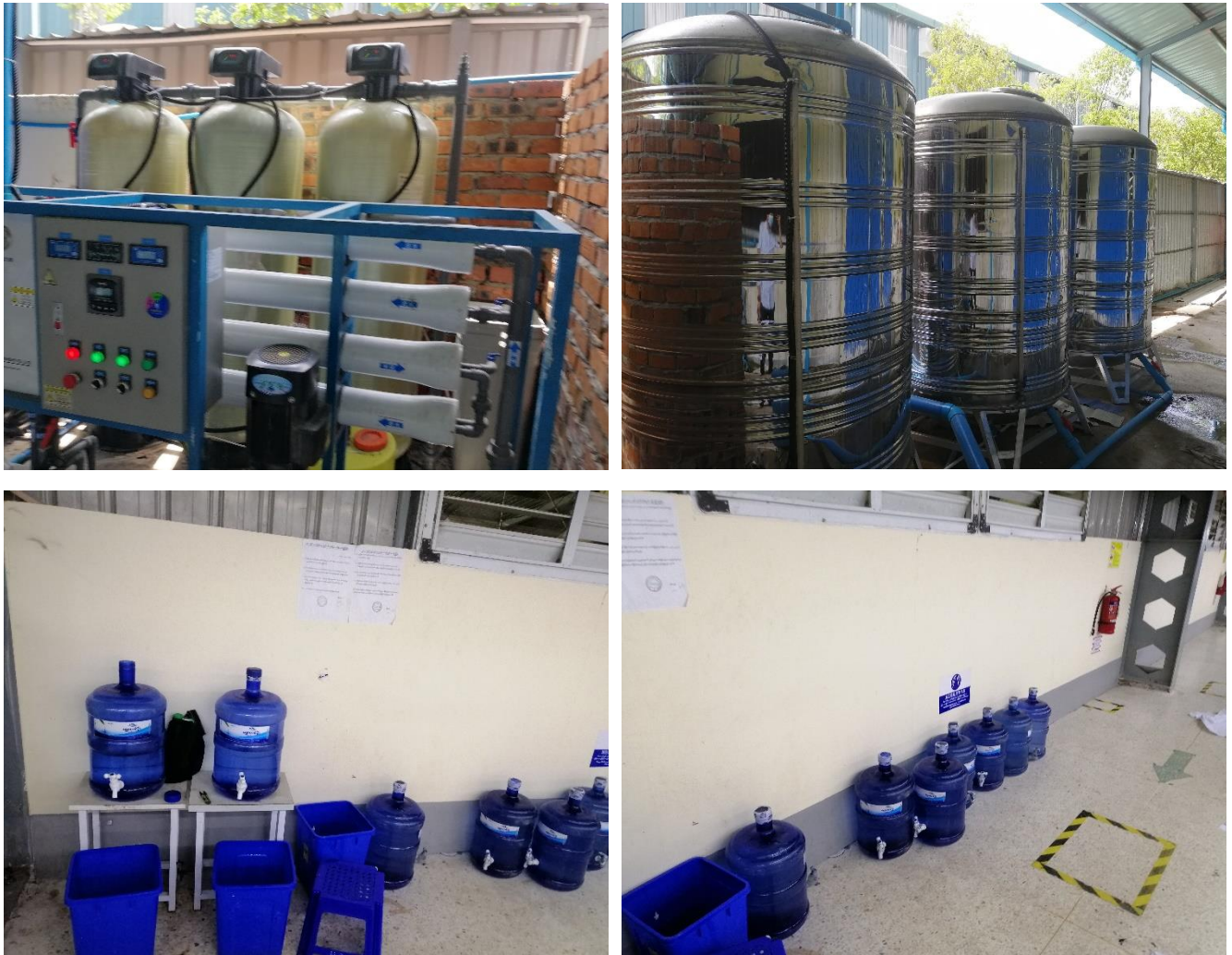
Figure 3-6 Water Storage Tank and Drinking Water Supply
