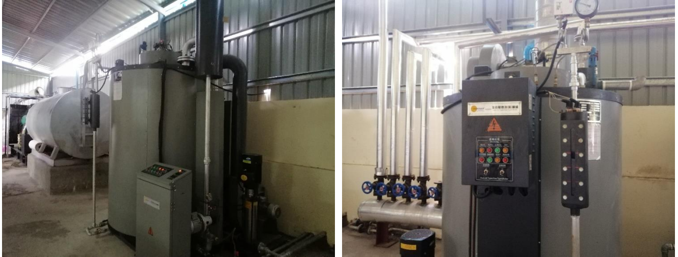
Figure 3-8 Boiler Usages of Sunrise (Myanmar) Fashion Company Limited
