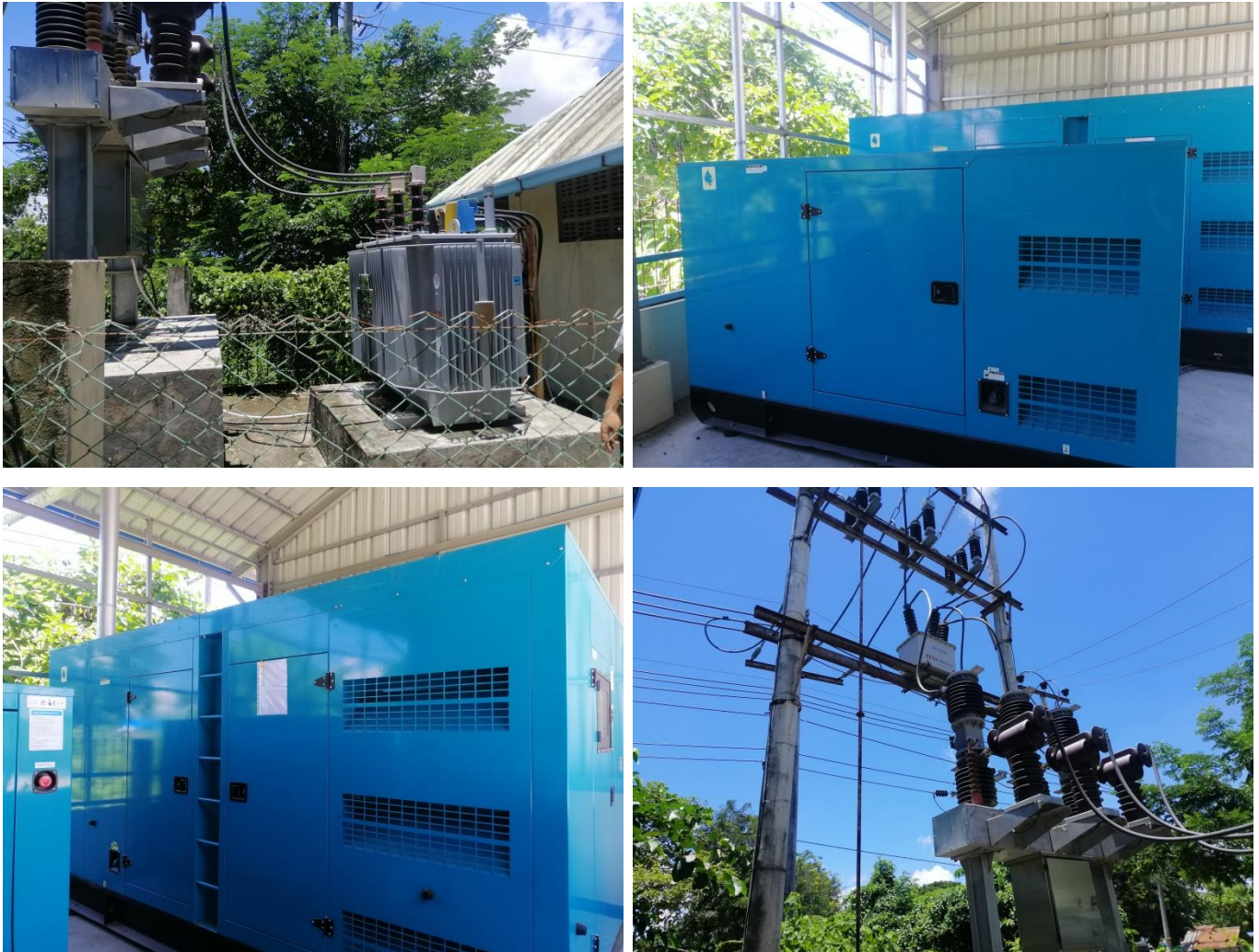
Figure 3-9 Electricity Facilities at Factory
